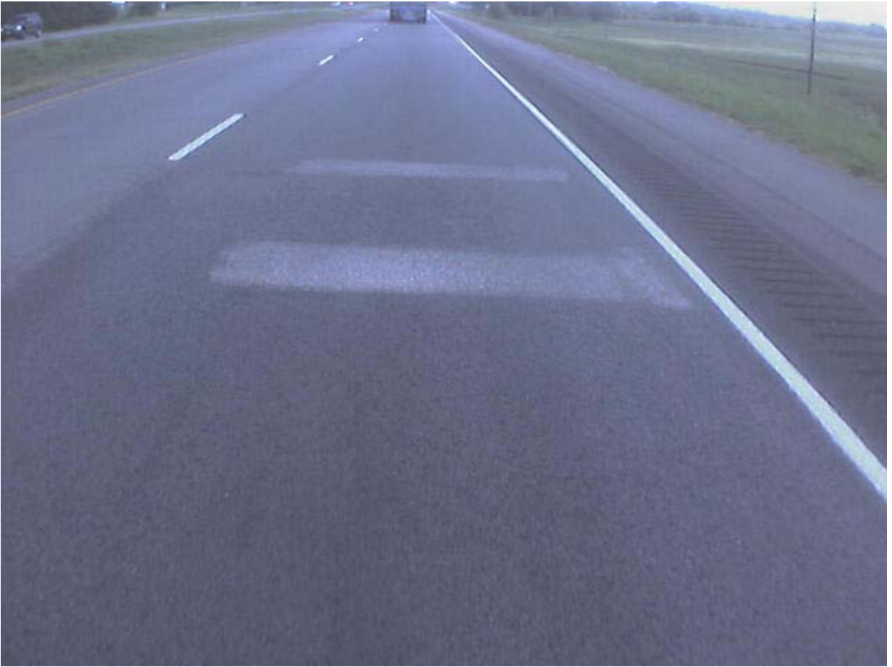
Figure A.2 Grind Spots along R1 Lane of US290 about 4147 ft from Start of Profile Survey
