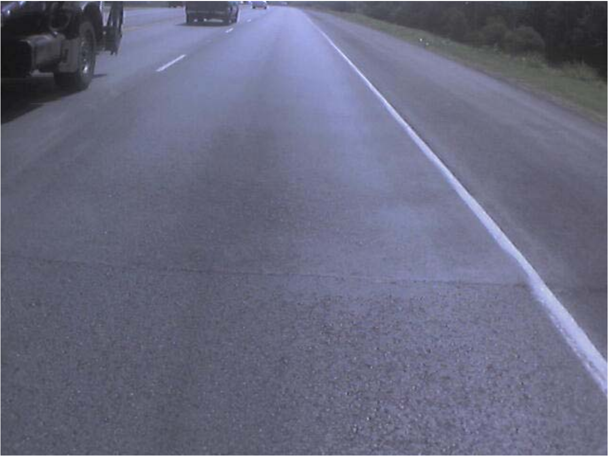
Figure A.4 Beginning of Overlaid Area on K1 Lane about 12,453 ft from Start of Survey
