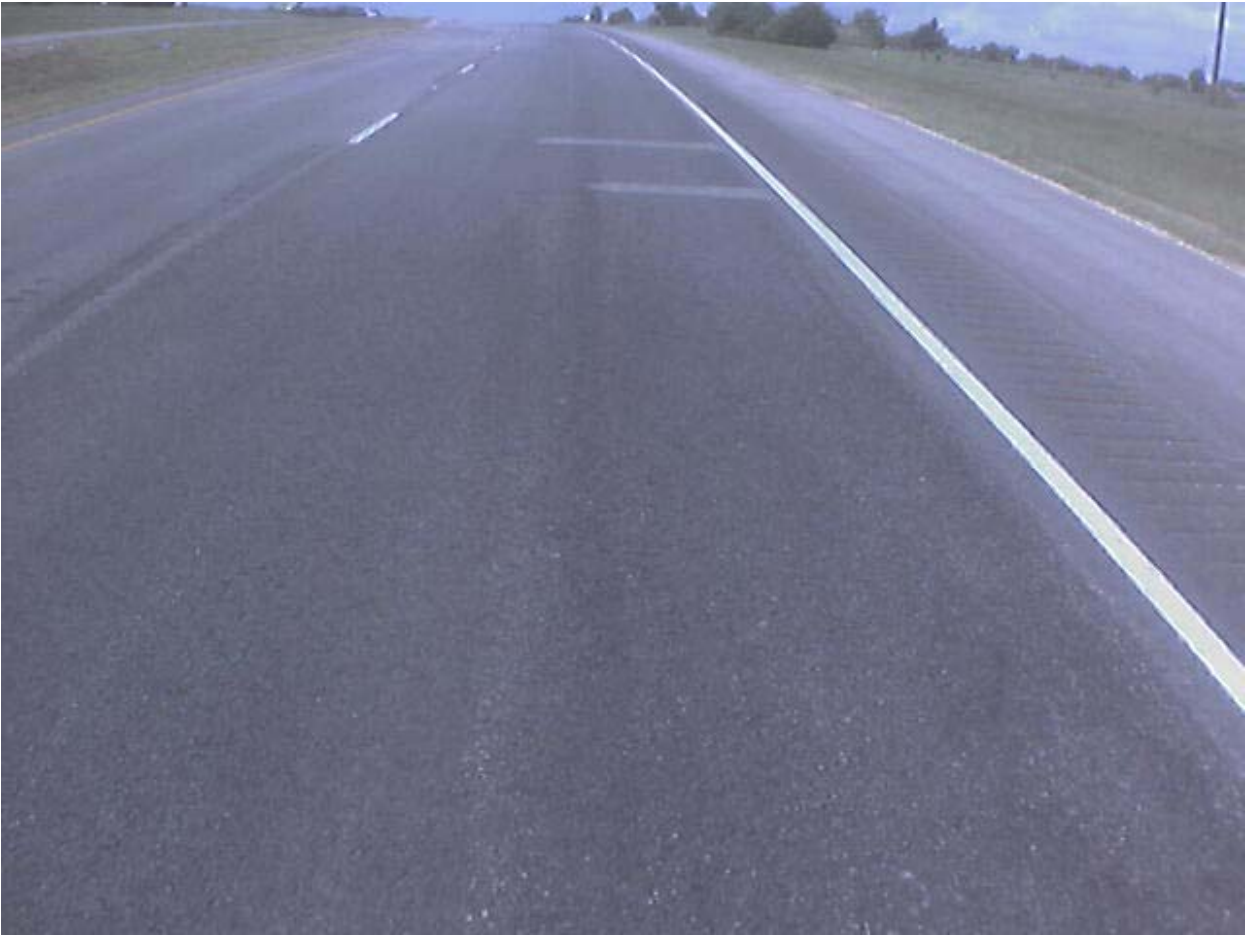
Figure A.3 Grind Spots along L1 Lane of US290 about 19,674 ft from Start of Survey
