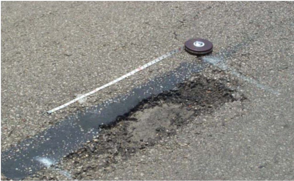
Figure 2.3 Pot Hole in Wheel Path of the Second 0.1 mile Section along Pearce Lane
