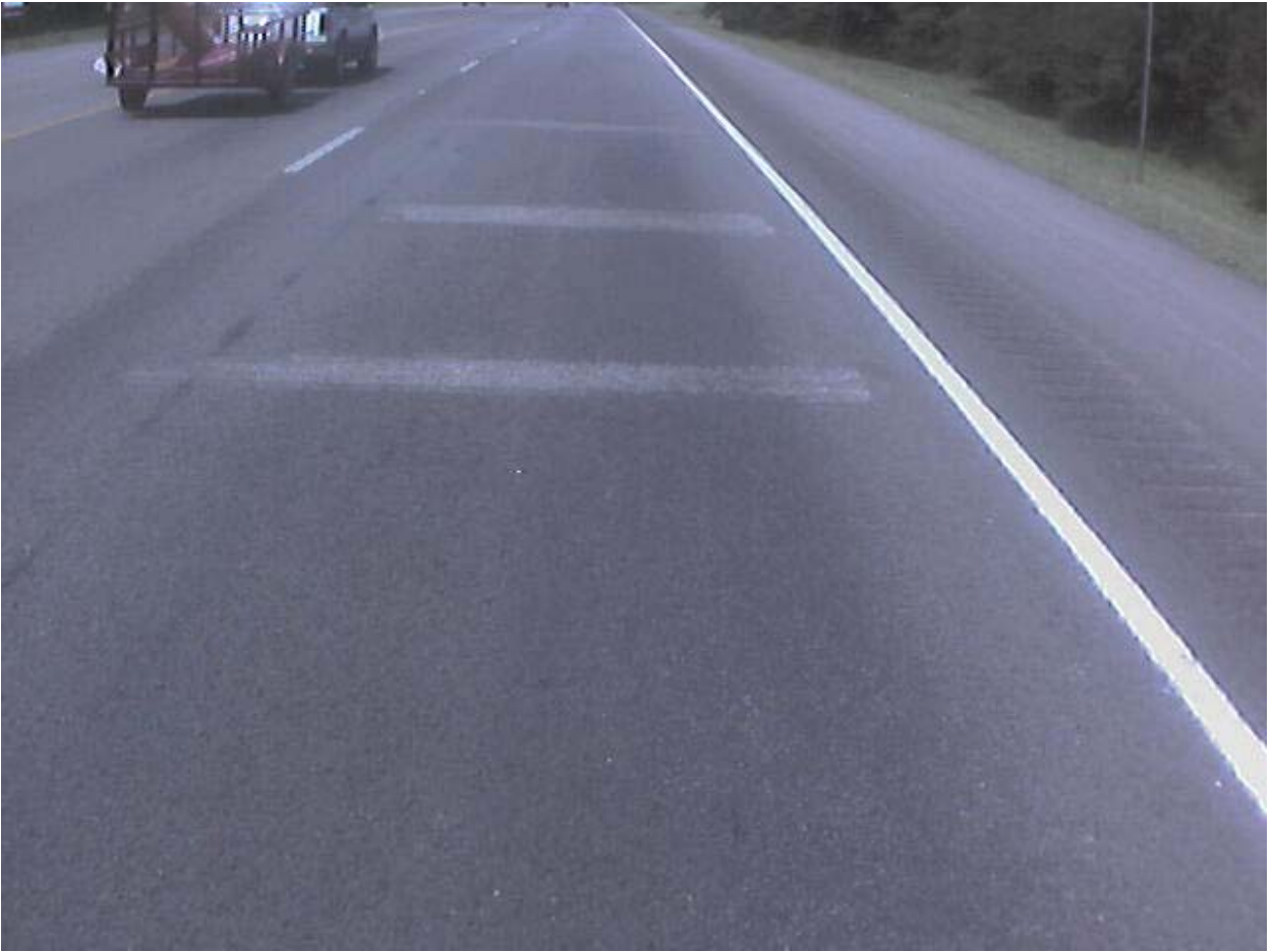
Figure A.5 Grind Spots along K6 Lane of US290 about 14,888 ft from Start of Survey
