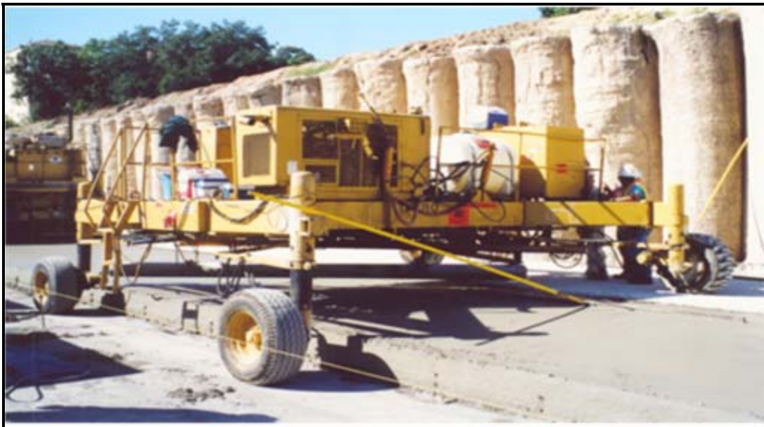
Figure 4. Finishing Tube with Motorized Carrier.
