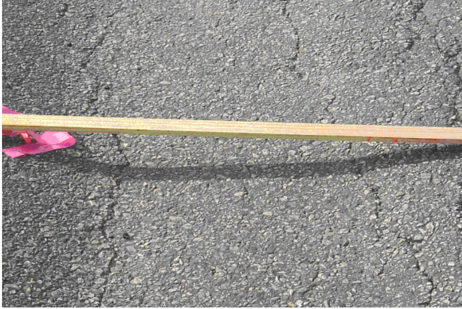
Figure 3.11 Deep Rutting at Decker Lane Location
