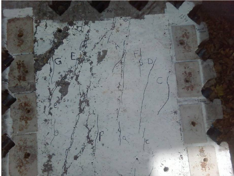
Fig. 6.2 Crack Pattern in PSFC Panel TAF-2
