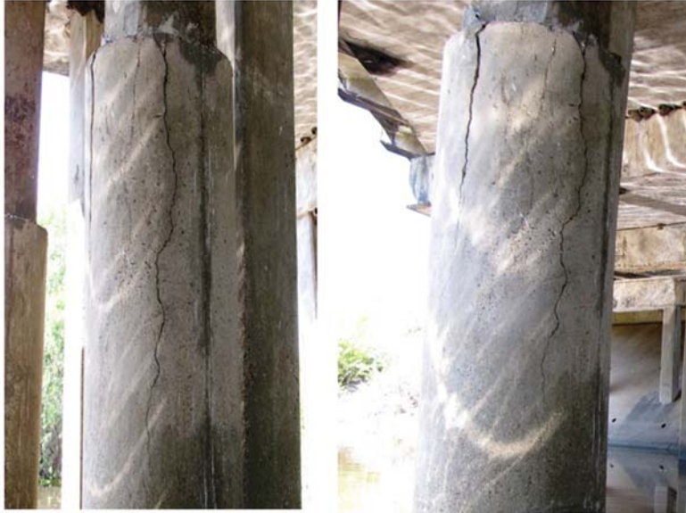
Figure 6. Cracked Collars Used to Repair Previous Spalling, TxDOT Beaumont District b. 1978.
