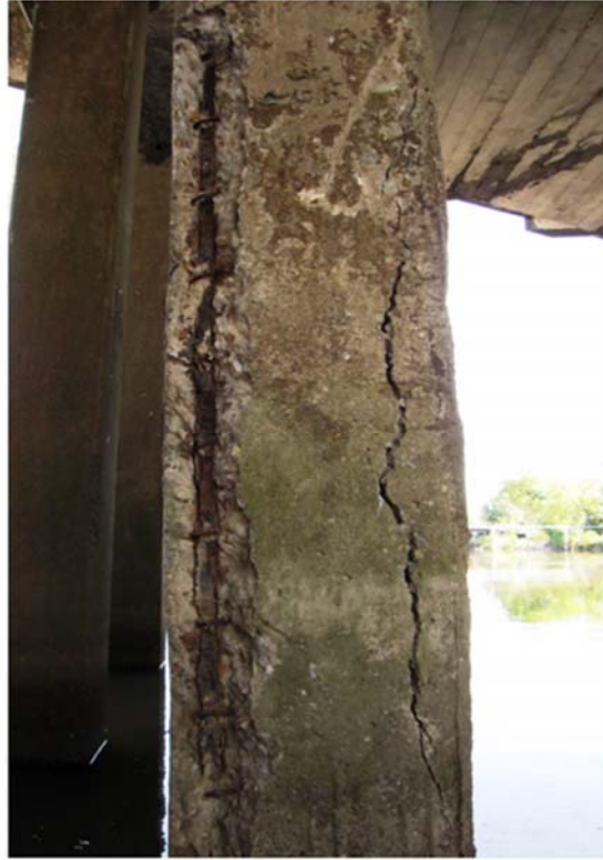
Figure 1. Deteriorated pile- cracked and spalling, TxDOT Beaumont District b. 1978.
