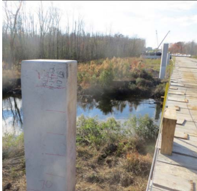
Figure 30. Successfully Driven Prestressed-CFRP Piles, Ozyildirim and Sharp (2013).
