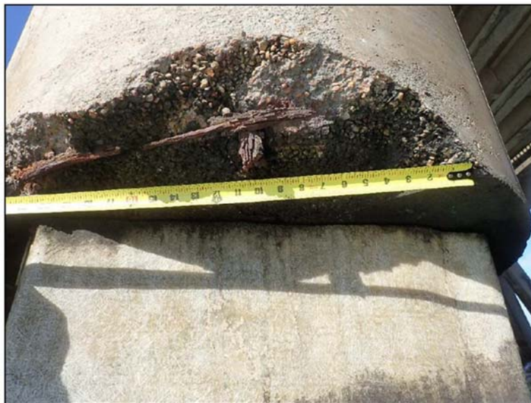
Figure 7. Spalling of Concrete Collar, Seawolf Parkway, TxDOT Houston District.
