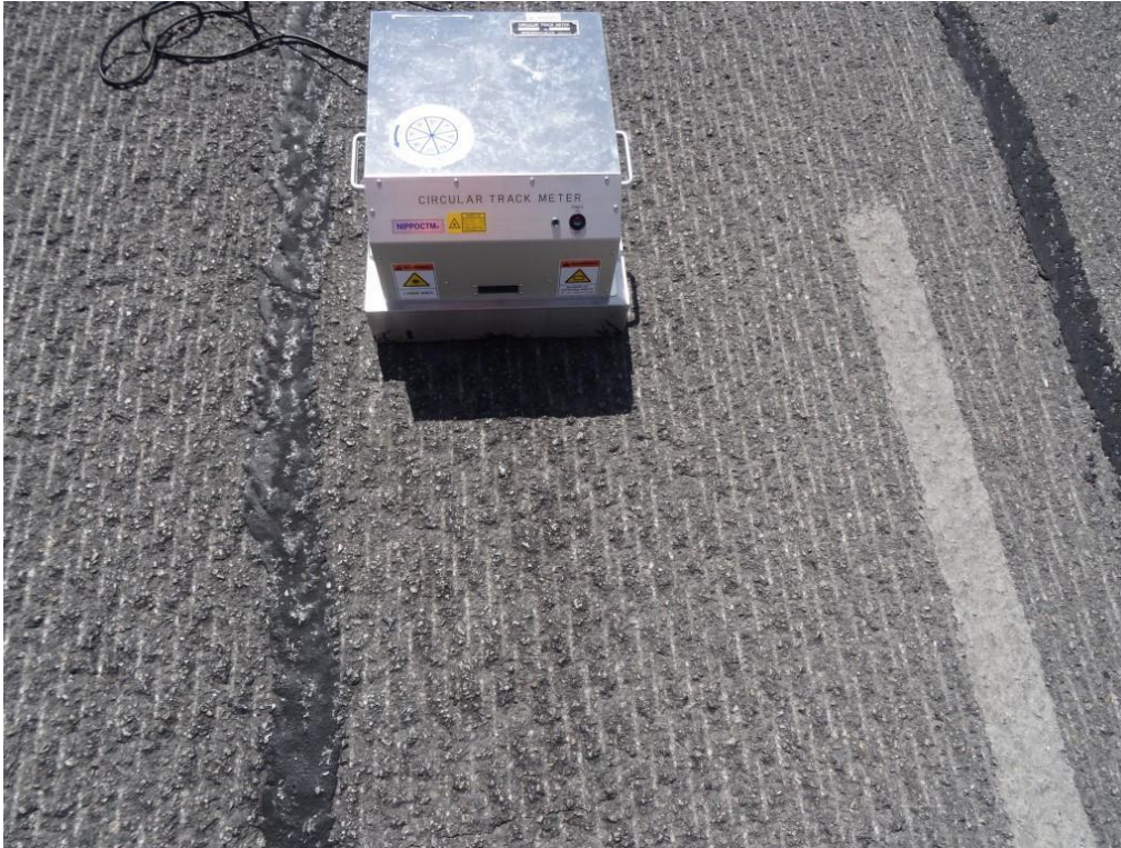
Figure 31. Photo taken from Wurzbach Parkway test site 18 months after the milling
