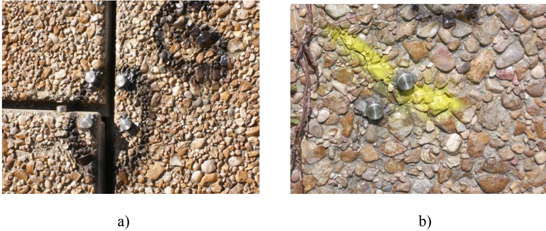
Fig. 5.23. Picture View of Demec Points on the Wall: a) for Wall Panel Displacement Monitoring and b) Crack Opening Monitoring (Project 3).
