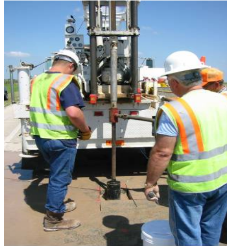
Figure 5.1 Field installation at Bryan District SPS-8 Site
