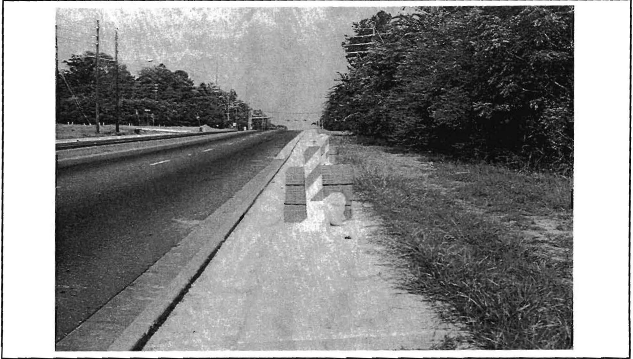
Figure C-5 Newly Widened Section is Tied into a Previously Widened Intersection in the Foreground
