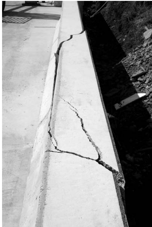
Figure 18. Failure mode for Test C.
