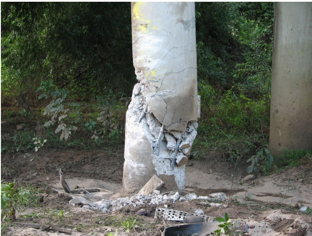
Figure 2.9. Truck Accident – IH-20 Bridge over Rabbit Creek, Longview, Texas.
