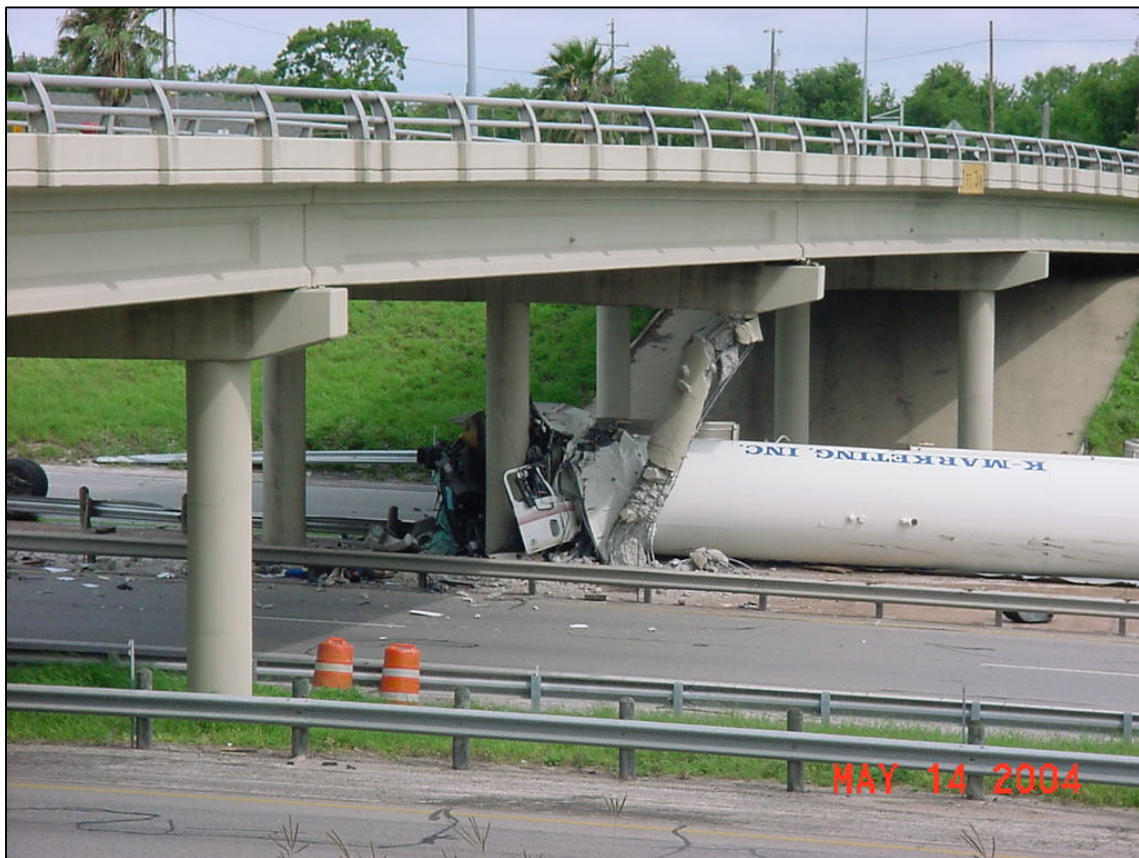
Figure 2.3. Truck Accident Tanchua Street Bridge over IH-37, Corpus Christi, Texas.
