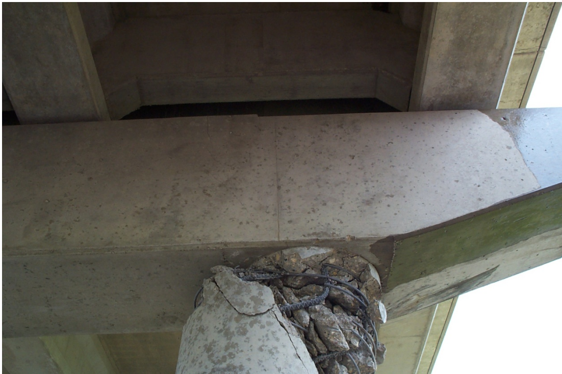
Figure 2.10. Truck Accident – IH-90 Bridge, #53812, Minnesota.
