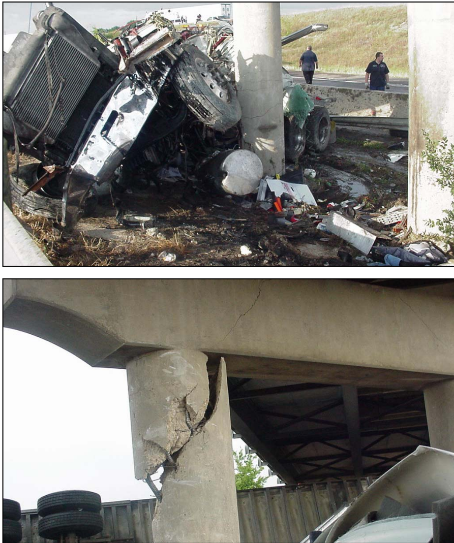
Figure 2.4. Truck Accident at Bridge at IH-35 and US-77, Red Oak, Texas.
