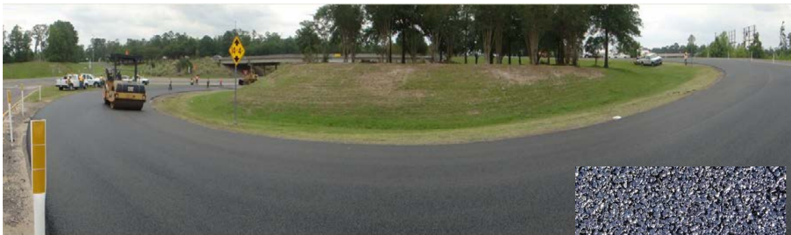
Very Thin, Fine-Graded PFC Placed on Cloverleaf Exit Ramp of US 59 Near Lufkin District Office. Maintenance needed a mix to address the numerous wet weather accidents occurring on this ramp.
