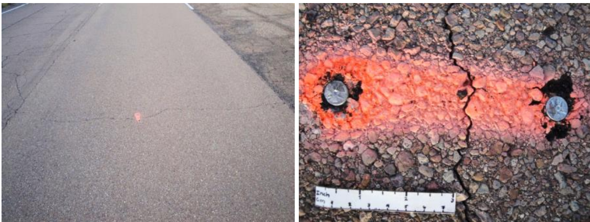
(a) Transverse Crack
