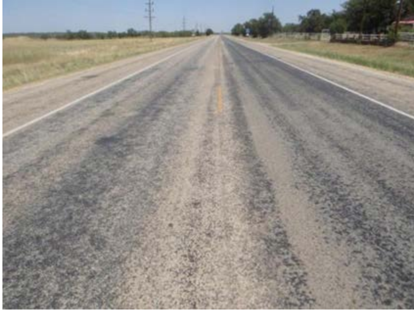
Figure 21. US 183 Bleeding Surface Treatment prior to PFC Surfacing.
