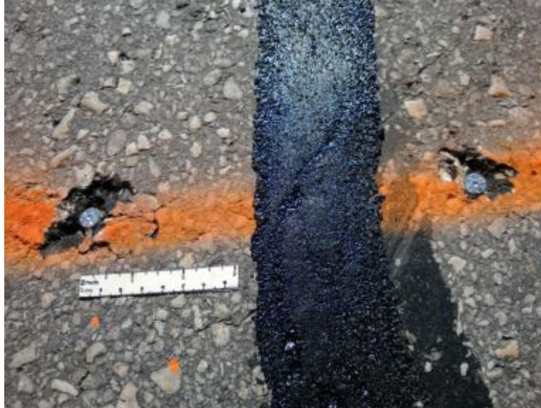
Figure 34. Reference Nails for Crack Measurements.
