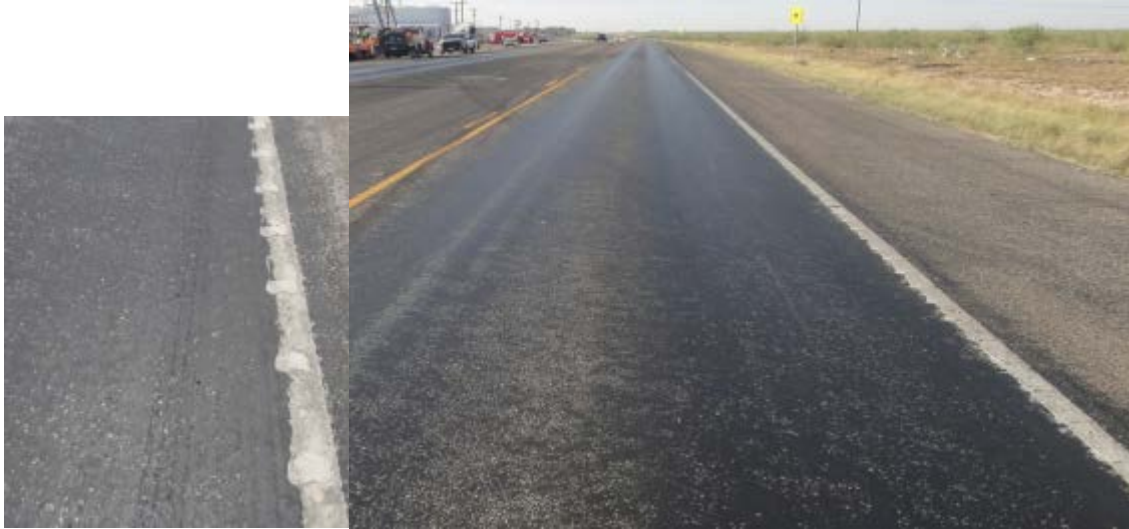
Figure 24. Pre-Existing Condition for Loop 338, Odessa District.
