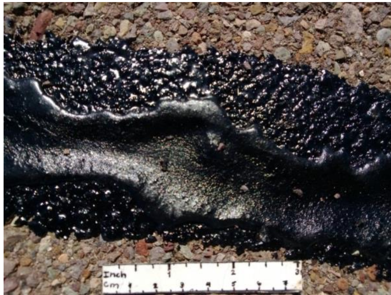
Figure 9. Non-Uniform Seal Caused by Sealant Flow.
