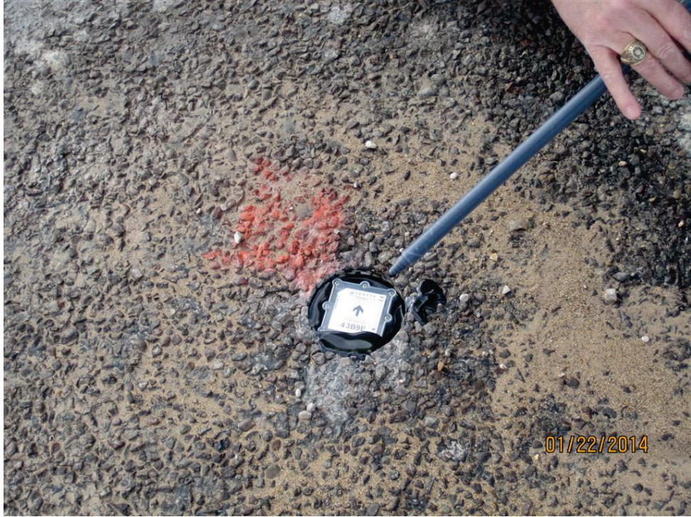
Figure 25. Wireless Sensor Installed in the Core.
