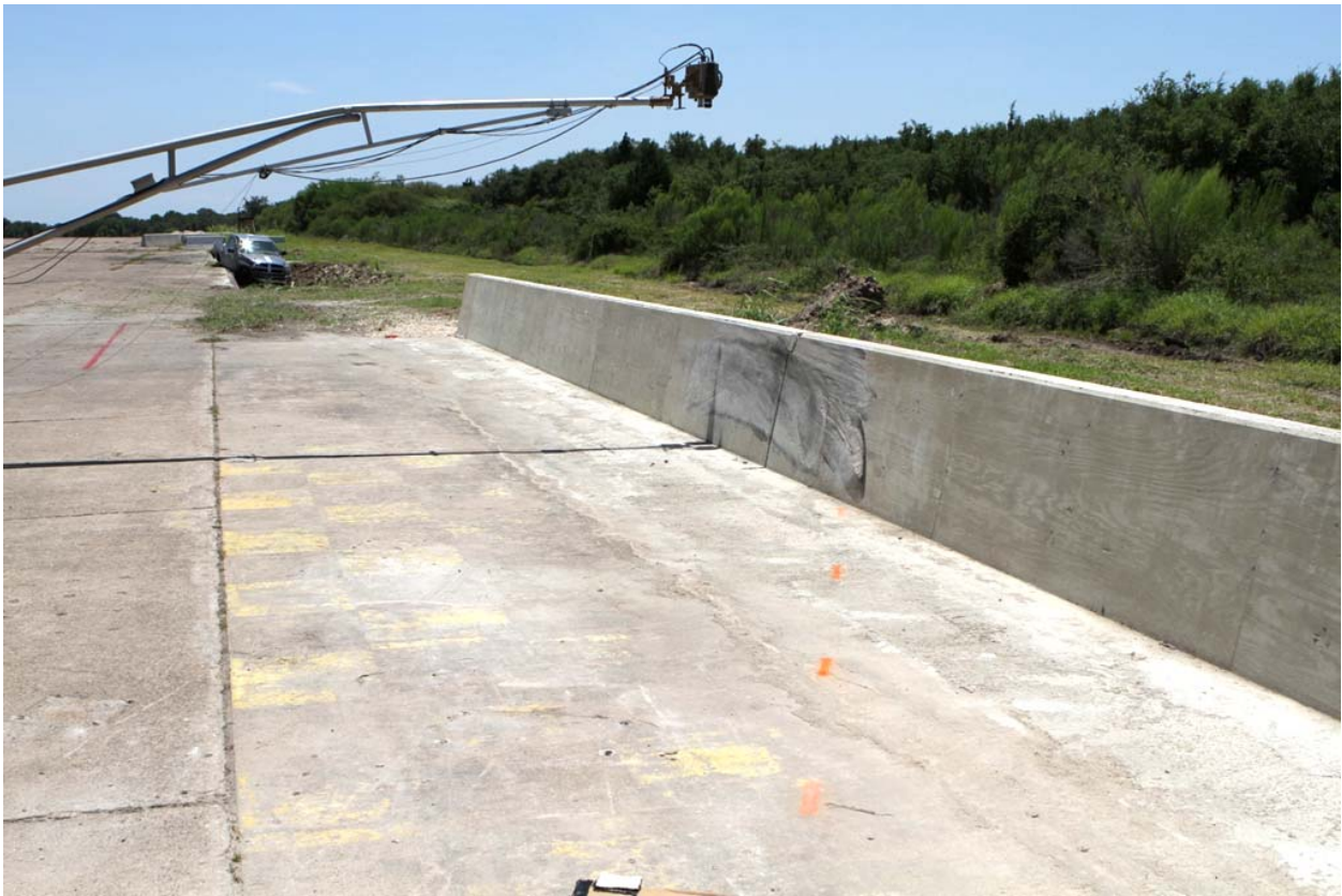
Figure 5.3. After Impact Vehicle Position for Test No. 420020-3.
