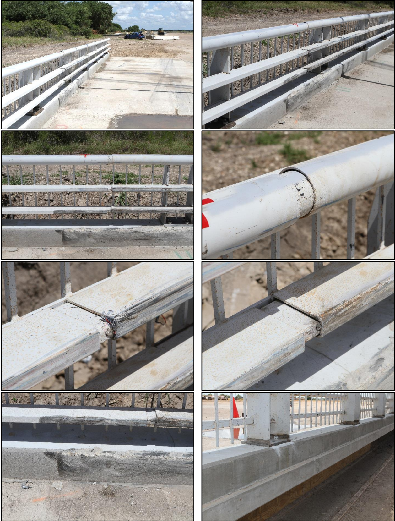
Figure 5-3. TxDOT Type C2P Bridge Rail after Test No. 490026-4-1.
