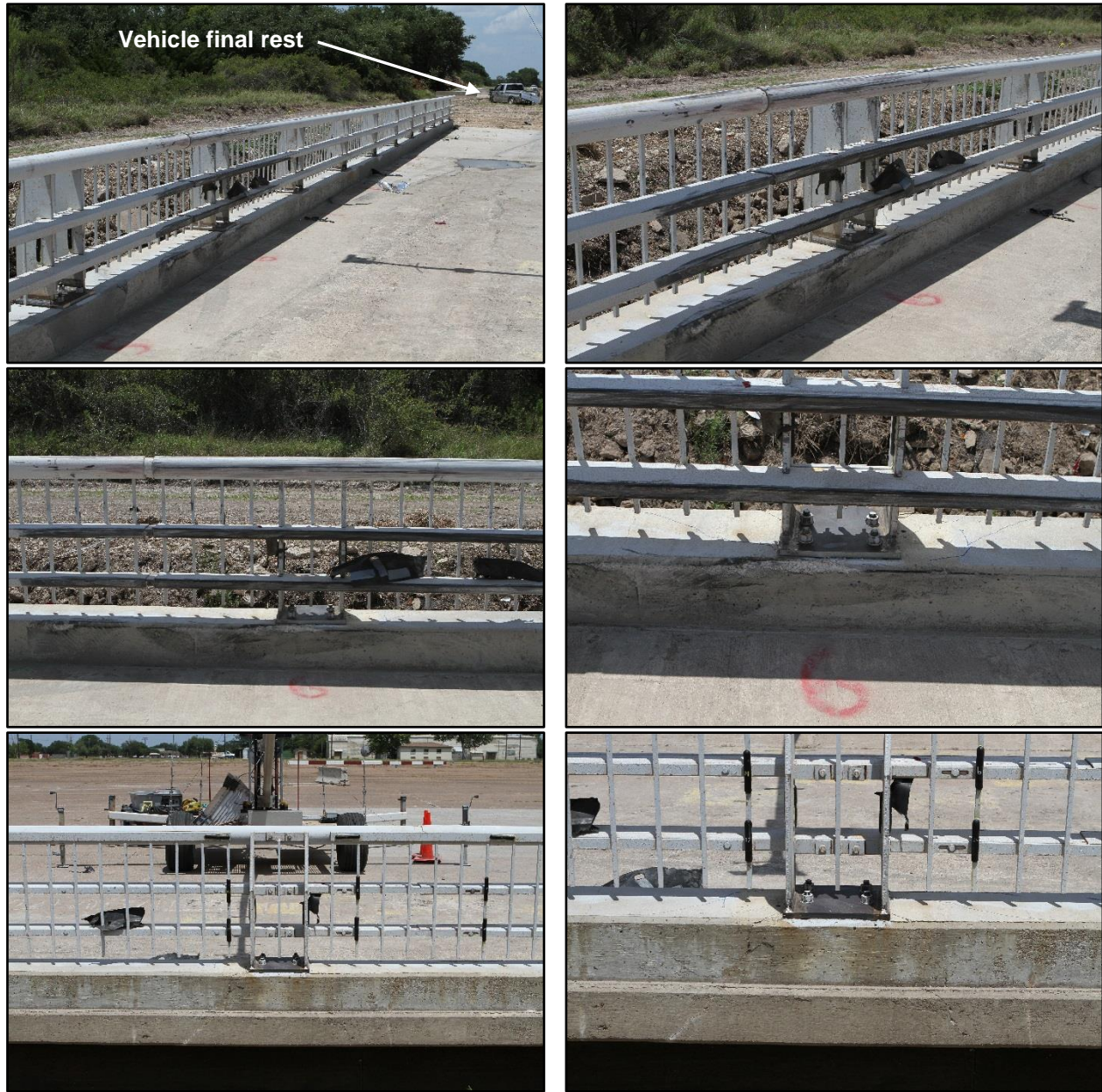
Figure 6-3. TxDOT Type C2P Bridge Rail after Test No. 490026-4-2.
