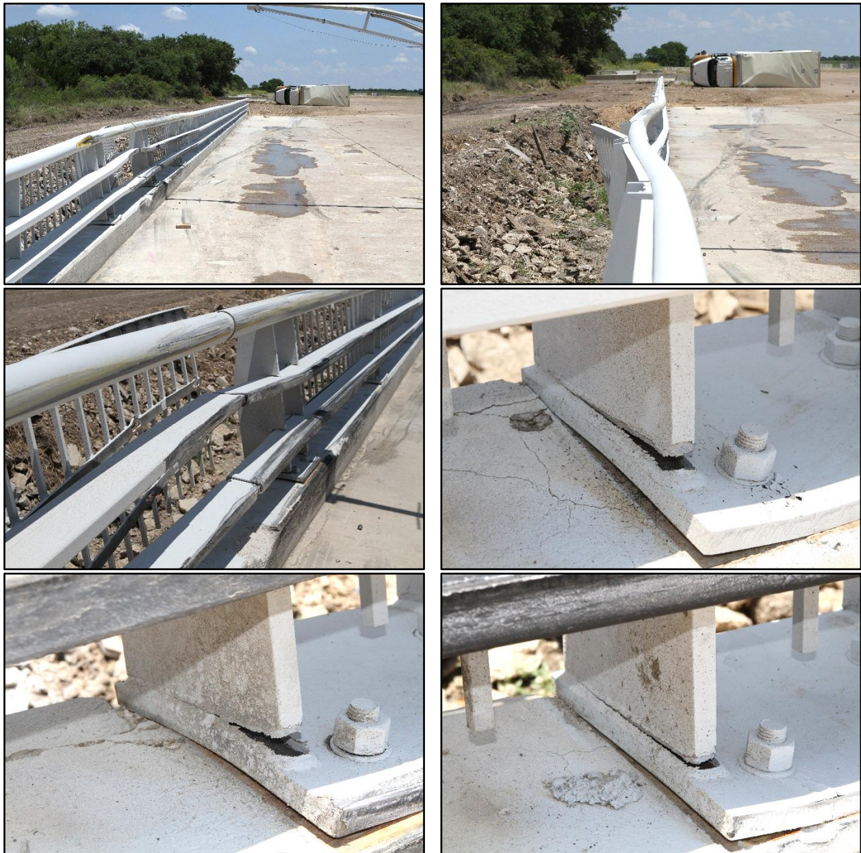
Figure 7-3. TxDOT Type C2P Bridge Rail after Test No. 490026-4-3.
