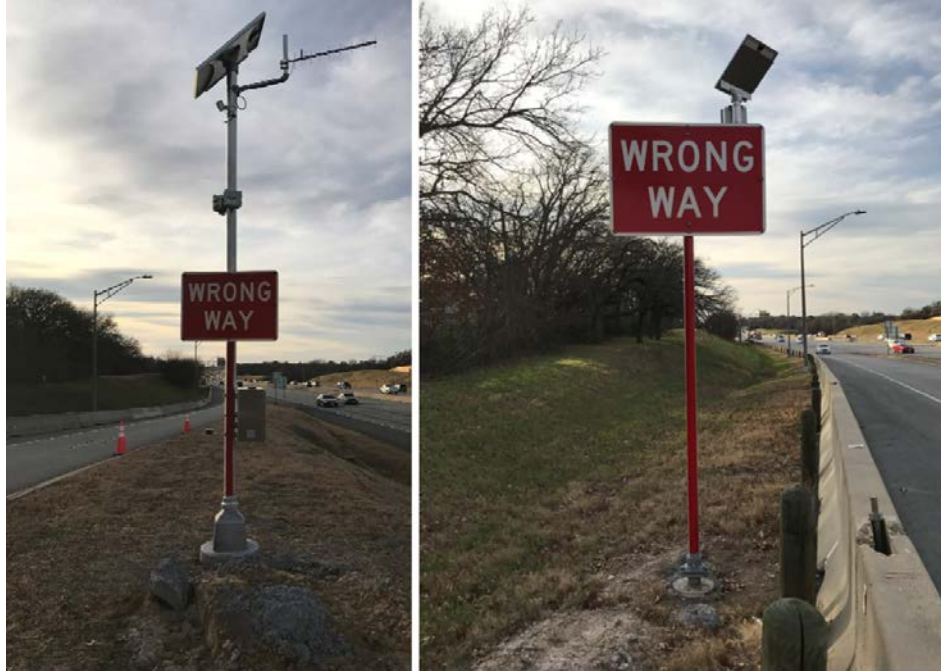
Figure 5. Solar-Powered LED Signs with Reflective Tape and Camera Monitoring System.
