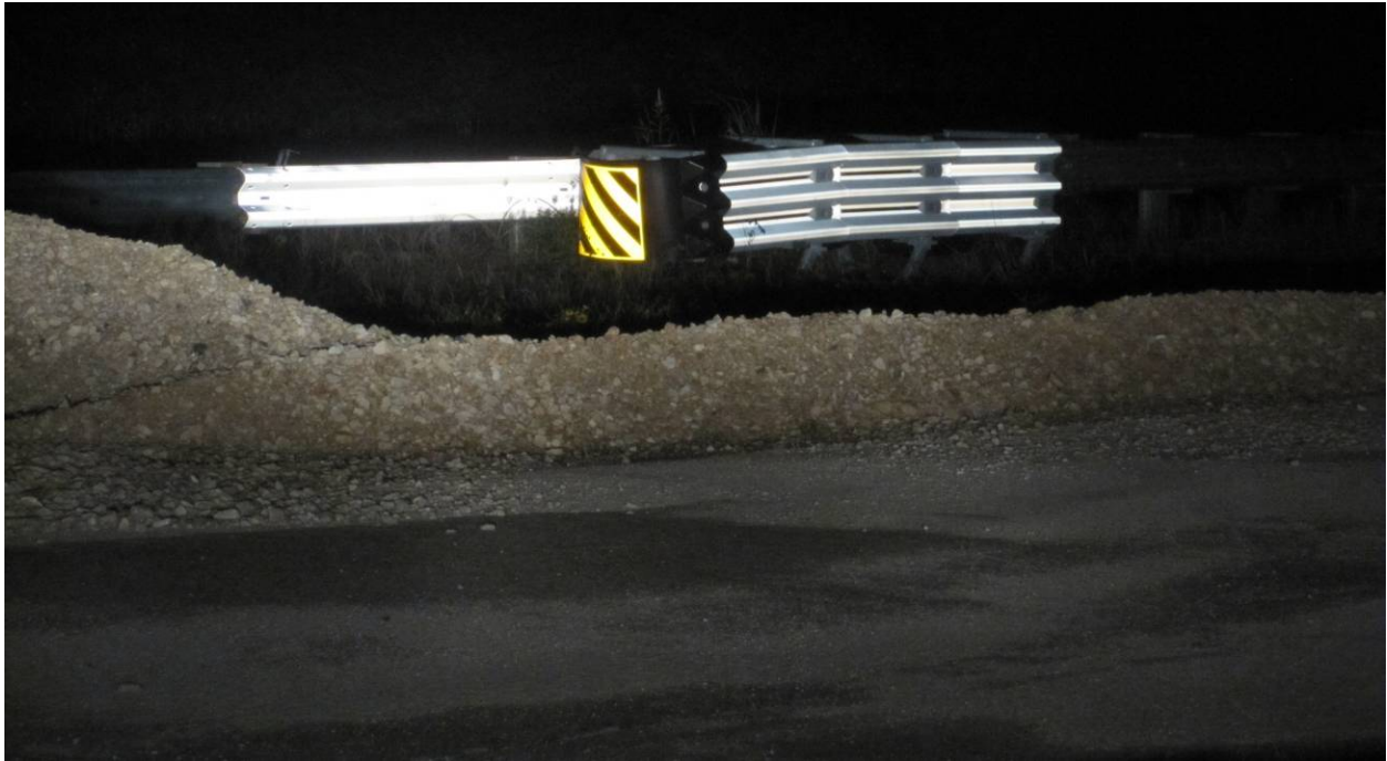
Figure 39. Retroreflective Powder Coated Guard Rail.
