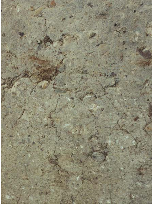
Figure 20. Microcracks in Cement-Treated Base Layer (18).
