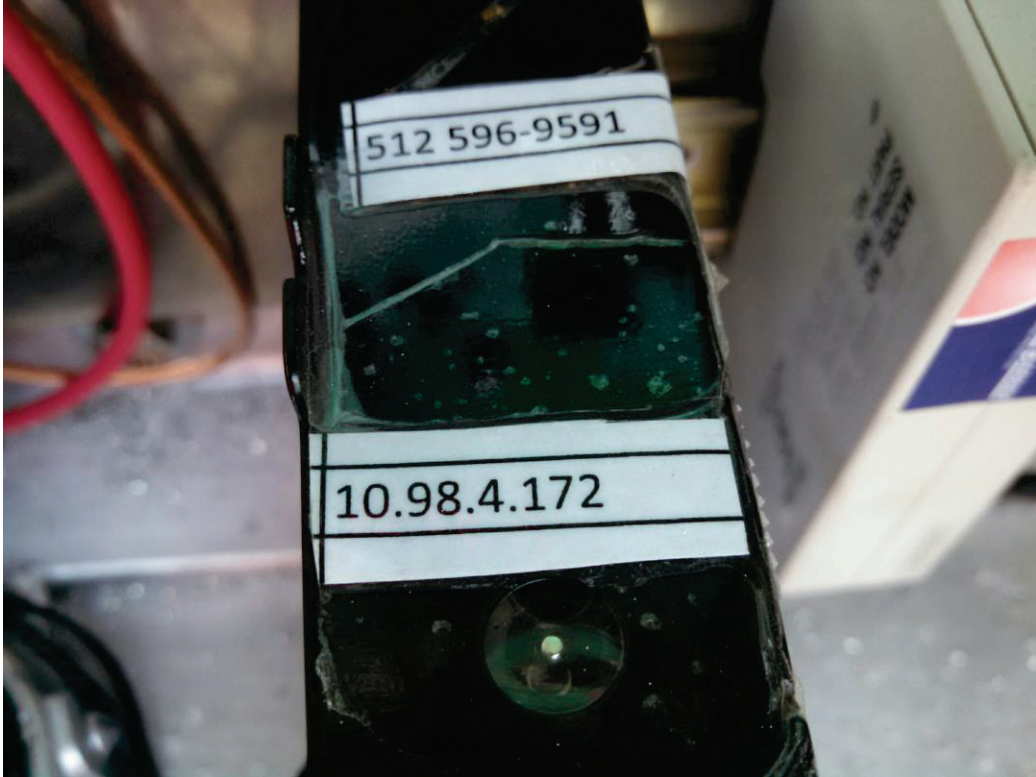
Figure 9. Wireless Modem Installed in Control Cabinet for Travel Time Sign Operation at Site 3.
