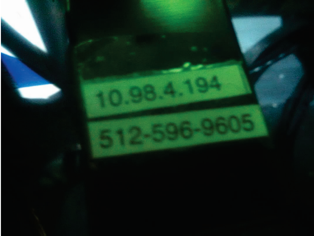
Figure 3. Wireless Modem Installed in Control Cabinet for Travel Time Sign Operation at Site 1.
