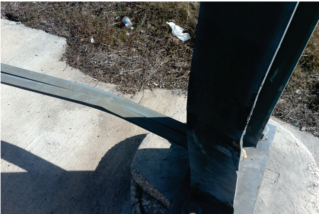
Figure 3. Damaged OSB Structure and Footing near Kyle.
