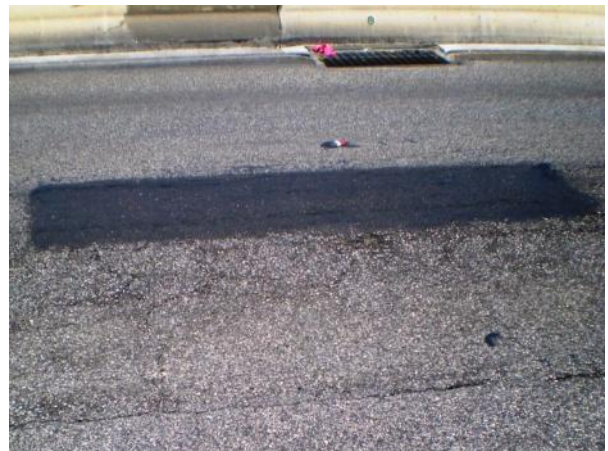
Figure 56. Patch 2/14-15 and 17 on Site IH10Fr.
