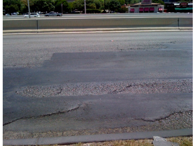
Figure 69. Shoving and Rutting Failure on Site IH10Fr.
