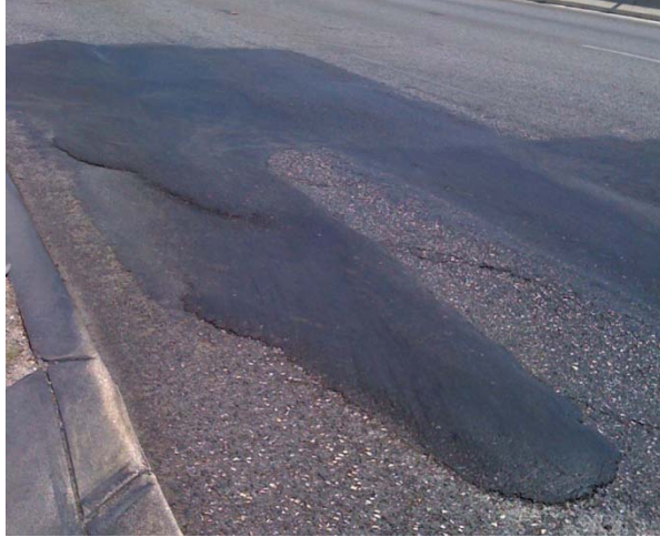
Figure 68. Shoving Failure at Site IH10Fr.
