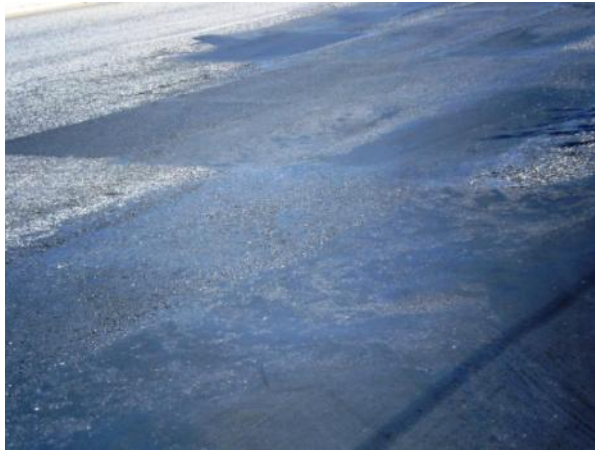
Figure 55. Various 2/10 Patches on Site IH10Fr.
