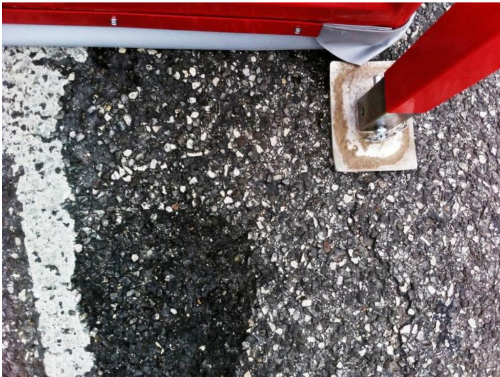
Figure 29. Close-up of Location of Patch 4 on IH410Fr-2.
