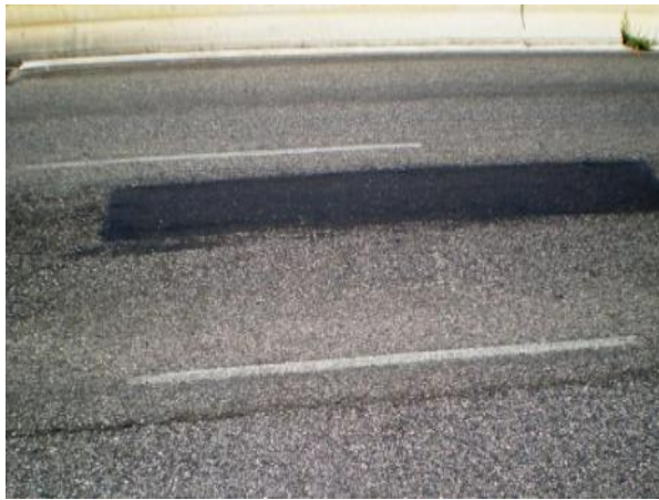
Figure 57. Patch 2/14-16 and 18 on Site IH10Fr.
