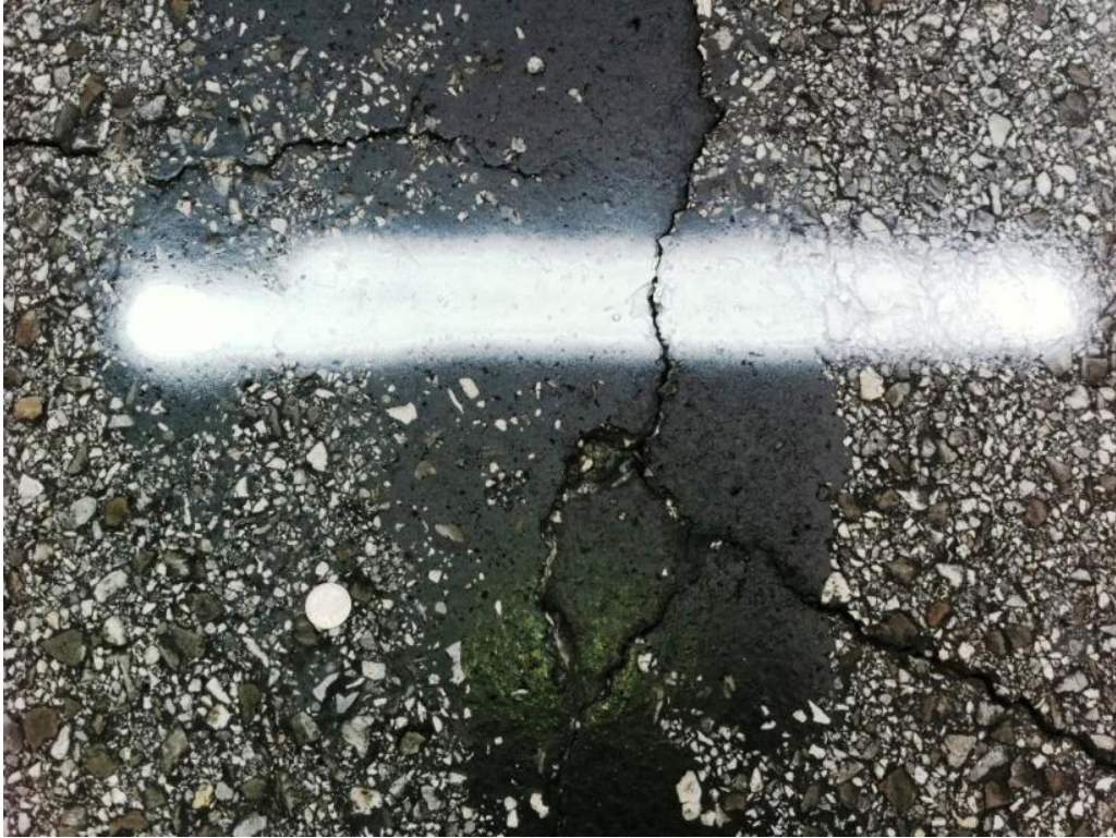
Figure 26. Close-up of Location of Patch 1 on IH410Fr-1.
