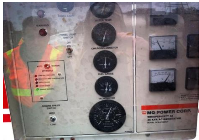
Figure 2. HeatWurx Gauges on Generator.
