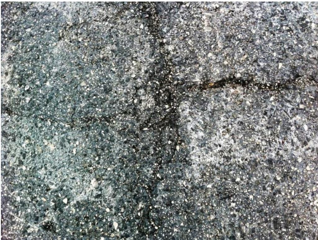
Figure 31. Close-up of Location of Patch 2/14-8 on IH10Fr-1.
