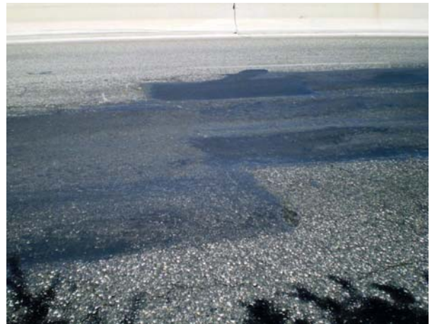
Figure 58. Various 2/14 Patches on Site IH10Fr.
