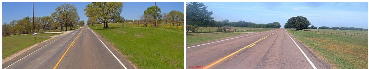
Figure 6. FM 1452 WB Surface Conditions: Before (Left) and After (Right) Seal Coat.
