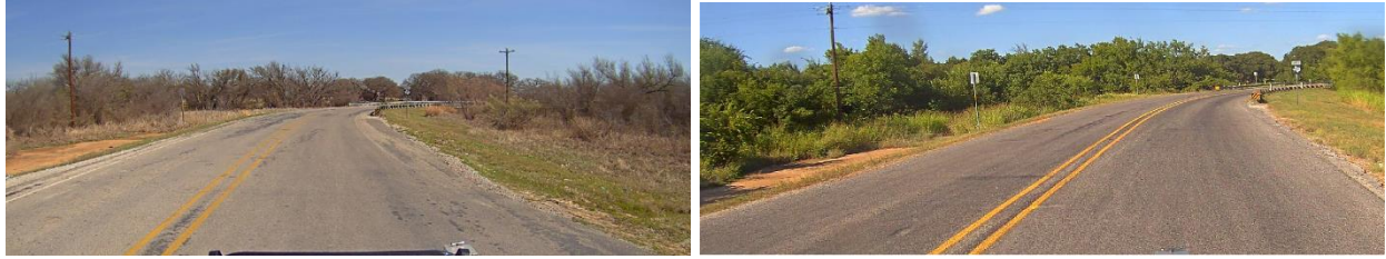
Figure 4. FM 587 EB Surface Conditions: Before (Left) and After (Right) Seal Coat.
