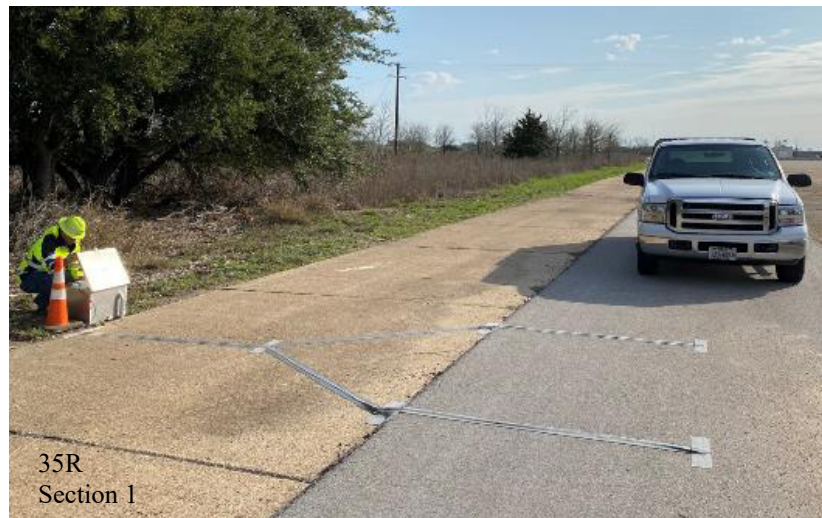
Figure 36. Sensor Checking, Testing, and Pre-calibration at the TTI Portable WIM Experimentation Test Site (Pocket-Tape).
