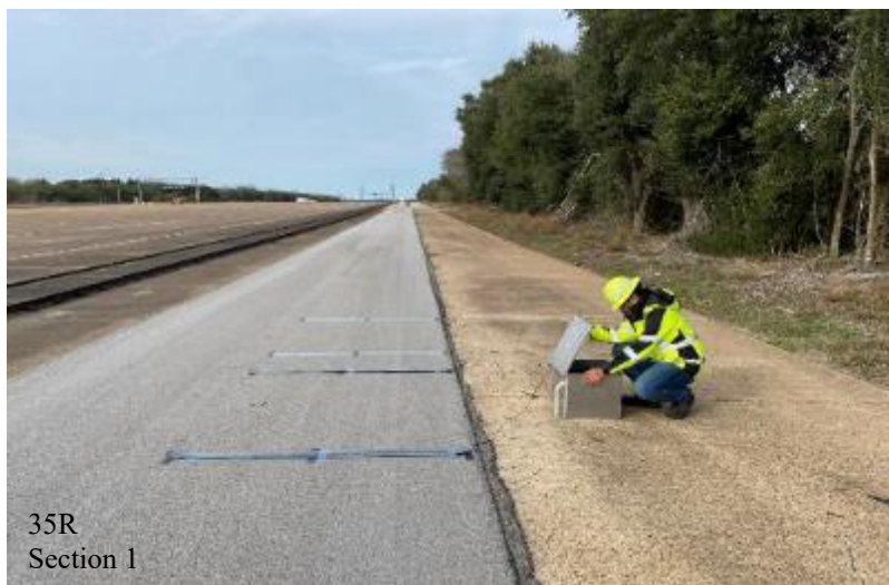
Figure 37. Sensor Checking, Testing, and Pre-calibration at the TTI Portable WIM Experimentation Test Site (Metal-Plates).
