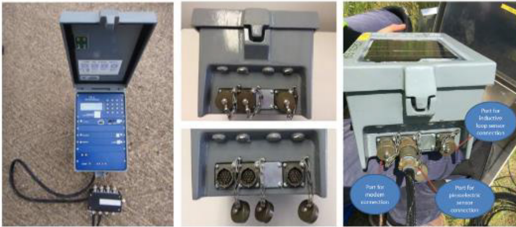
Figure I-1. Three-Channel TRS Portable WIM Unit. (Piezo-electric Channel (2 nd channel) = 8 Sensors or 4-Lanes).
