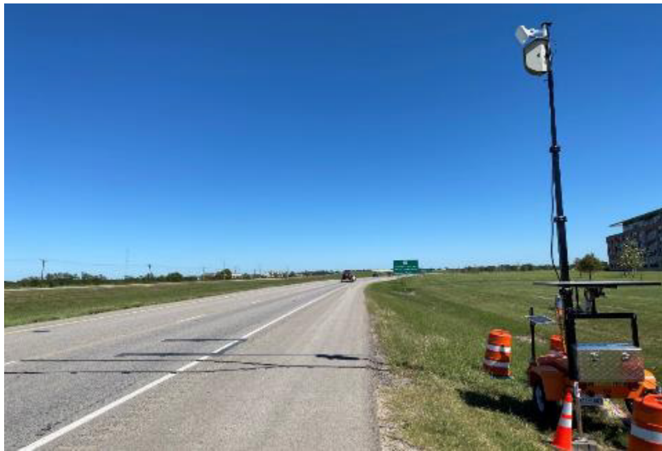
Figure 41. Portable WIM Demo-Monitoring Testing Station in SH 21 (EB), Bryan District.
