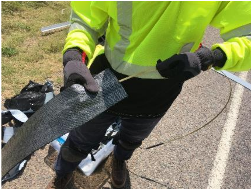
Figure 37. Inserting the Piezoelectric Sensors into the Pocket Tapes.
