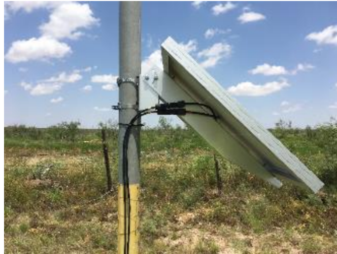
Figure 48. Solar Panel Mounted on a Pole.
