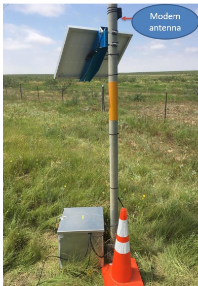
Figure 59. Attached Modem Antenna.
