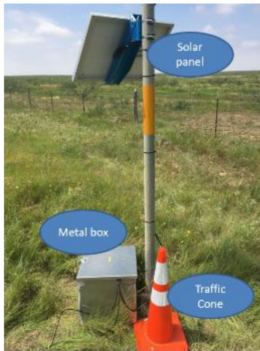
Figure 51. Metal Box, Traffic Cone, and Mounted Solar Panel.
