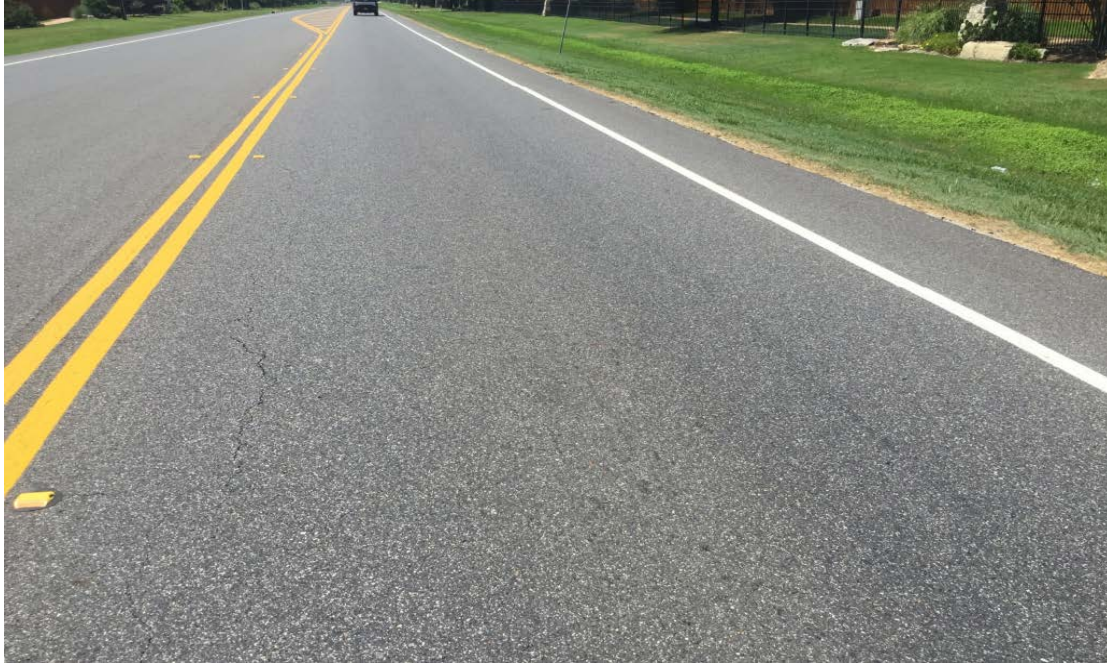
Figure 65. Longitudinal Crack on FM 1463_S4 Test Section.
