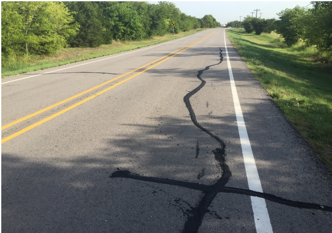
Figure 64. Transverse Crack and Longitudinal Crack on FM 3549 Test Section.
