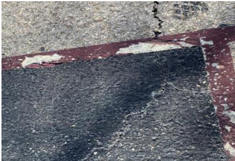
Figure 36. Crack Sealing Failure on SH 21.
