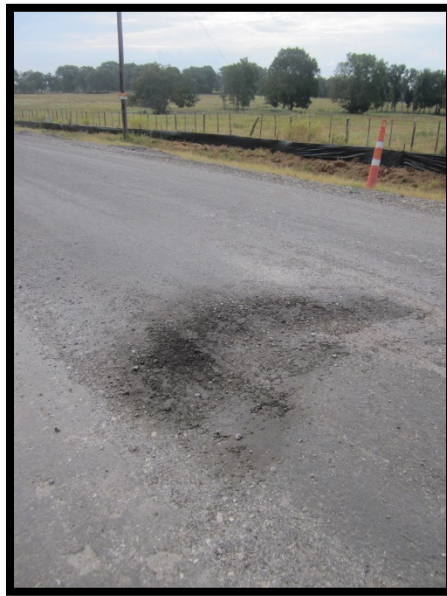
Figure 47. Localized Failure Due to Excessive Water at Location of Disconnecting FDR Train.
