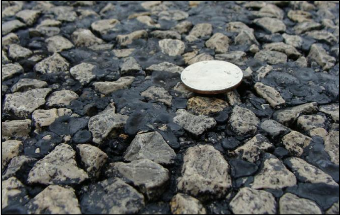
Figure 7. Wheel Path Texture Close-up on US 283 Two Years after Seal Coat Placement.
