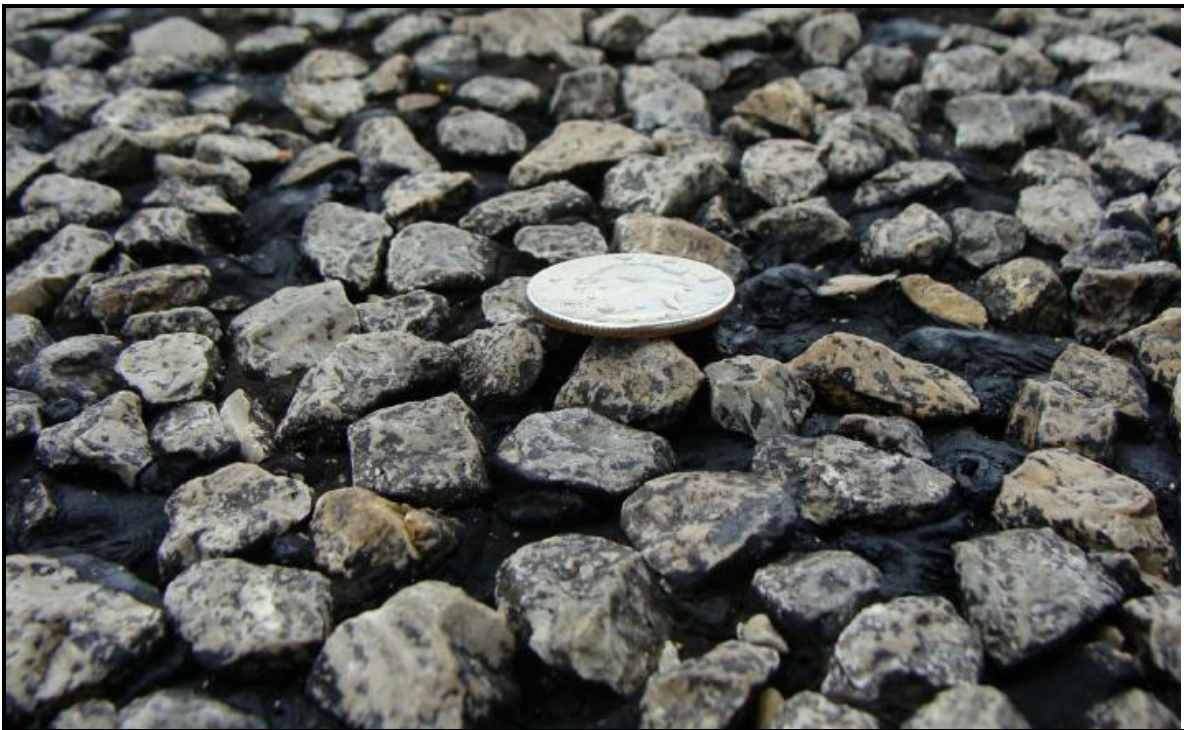
Figure 8. Between Wheel Path Texture Close-up on US 283 Two Years after Seal Coat Placement.
