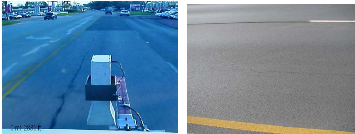
Figure 20. Before and After Photos of an Area Showing Fine Longitudinal Cracking.
