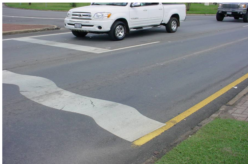
Figure 21. Mix Instability at One Stop Sign Associated with Construction Problems.
