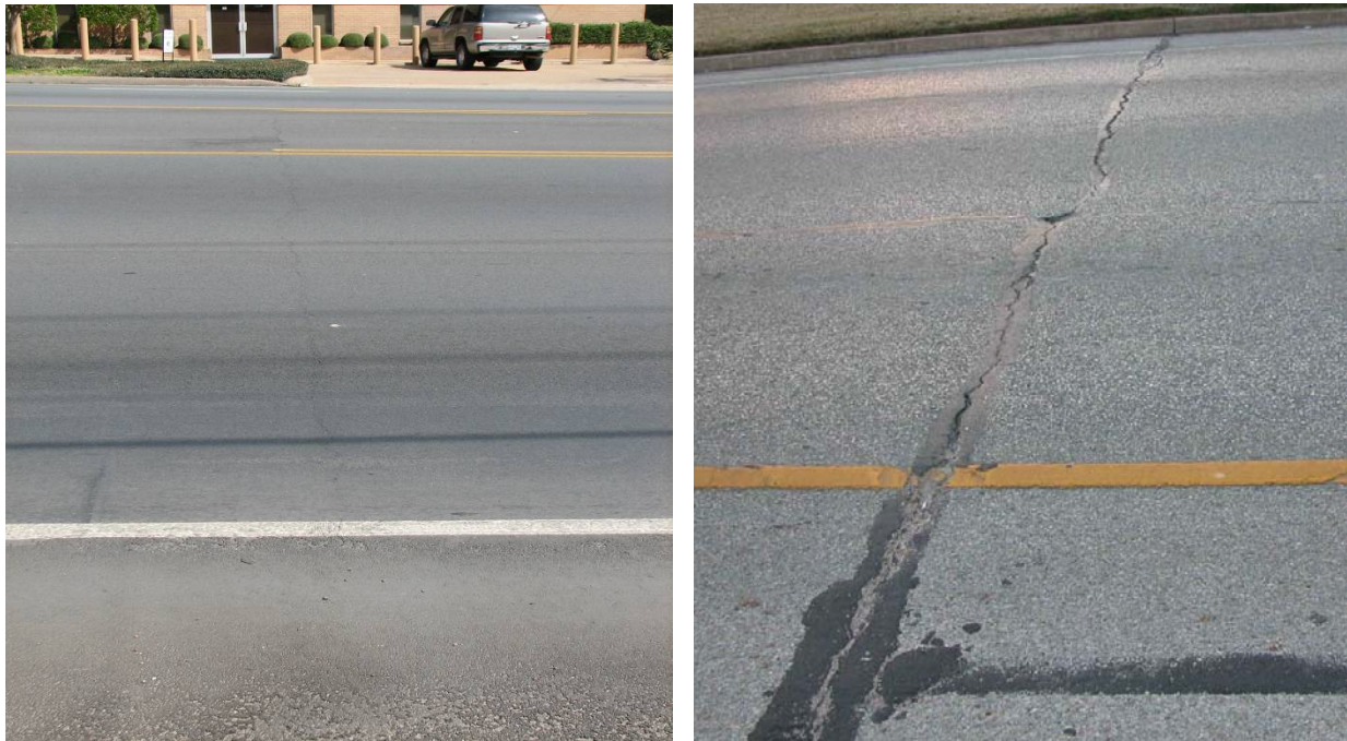
Figure 19. Low Severity Reflection Cracking after 1 Year – Original Condition on Right.
