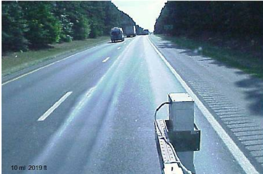
Figure 3.40. Rutting for 2-miles in Westbound Direction (Atlanta-Fine SMA).
