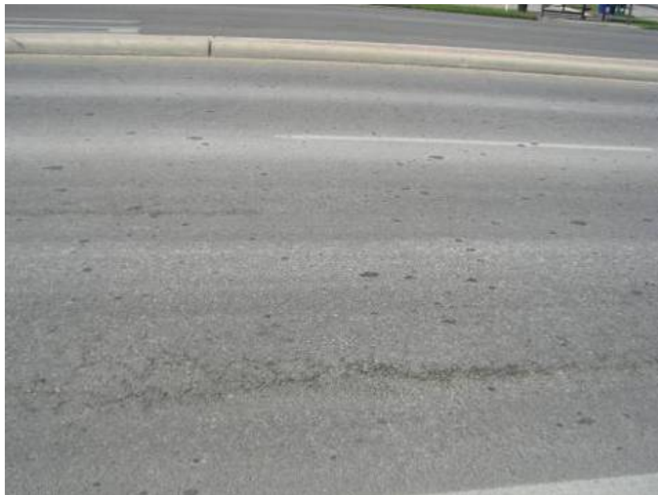
Figure 3.6. Evidence of Longitudinal Cracking Appearing in Both WMA and HMA Sections.
