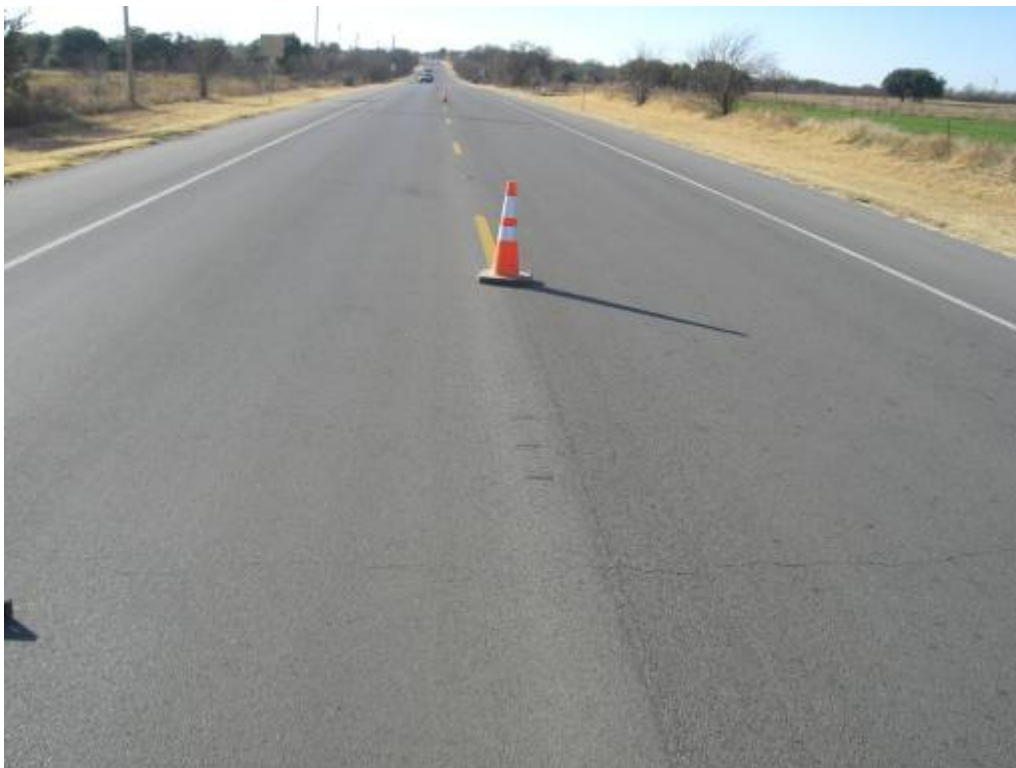
Figure 3.35. Transverse Cracking in both HMA and WMA Sections of SH 251.
