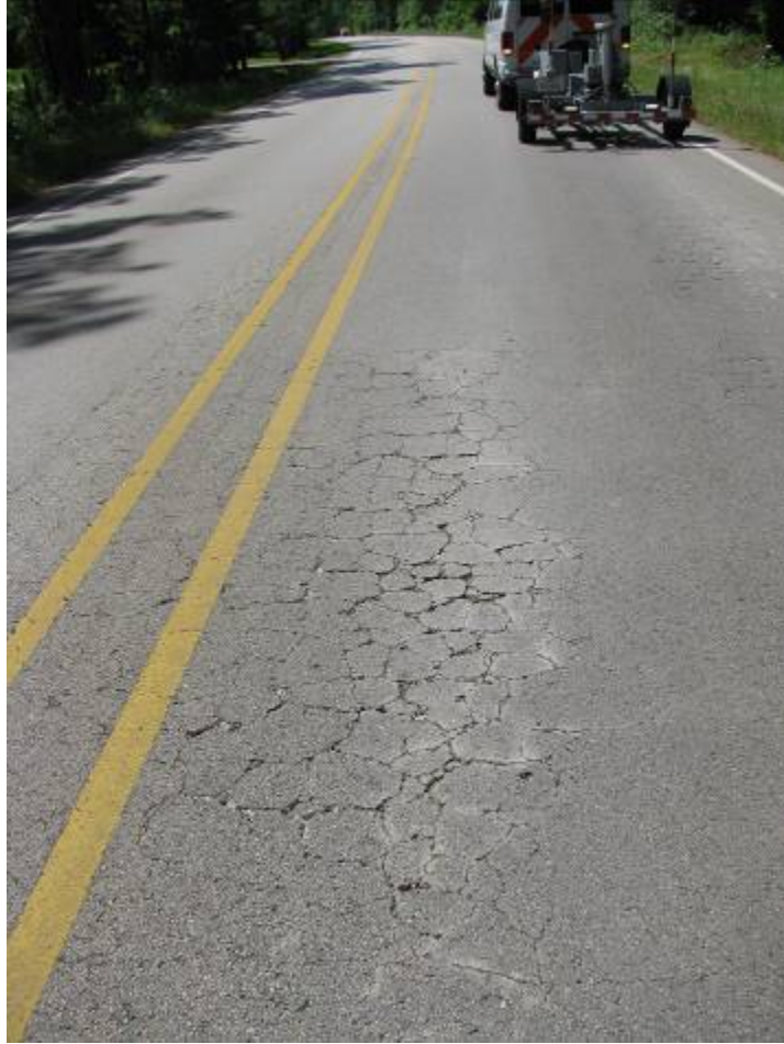
Figure 3.17. Alligator Cracking at South End of Project.
