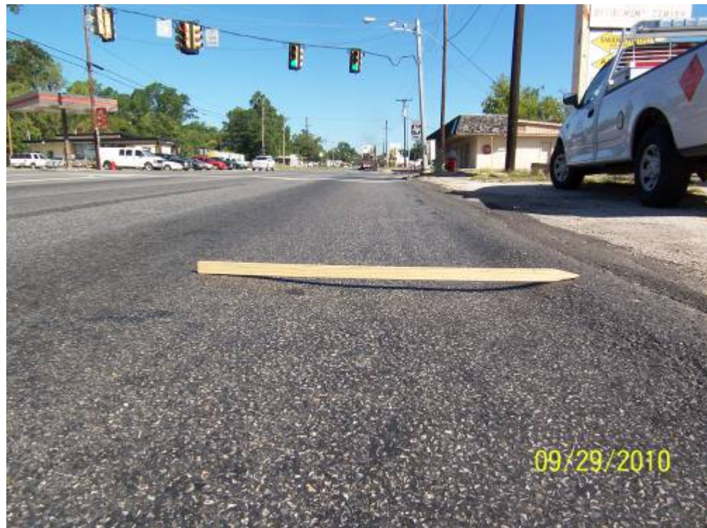
Figure 3.42. Rutting Intersections on US 96.
