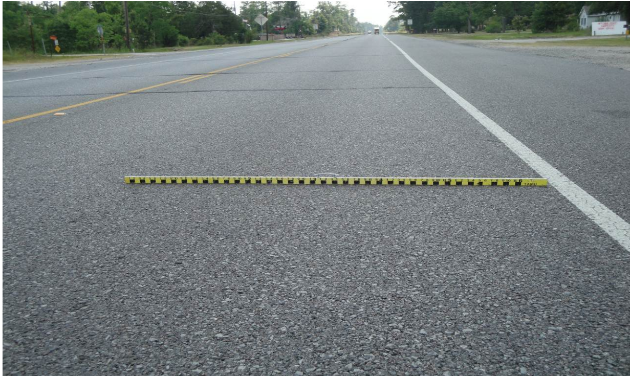
Figure 3-13. Rut Measurement on SH 12.
