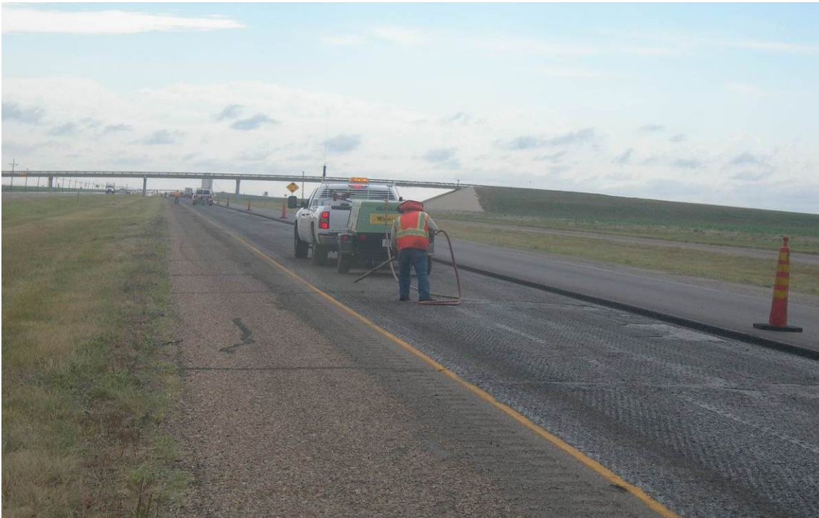
Figure 6-1. Existing Pavement Condition of IH 40 Test Sections.
