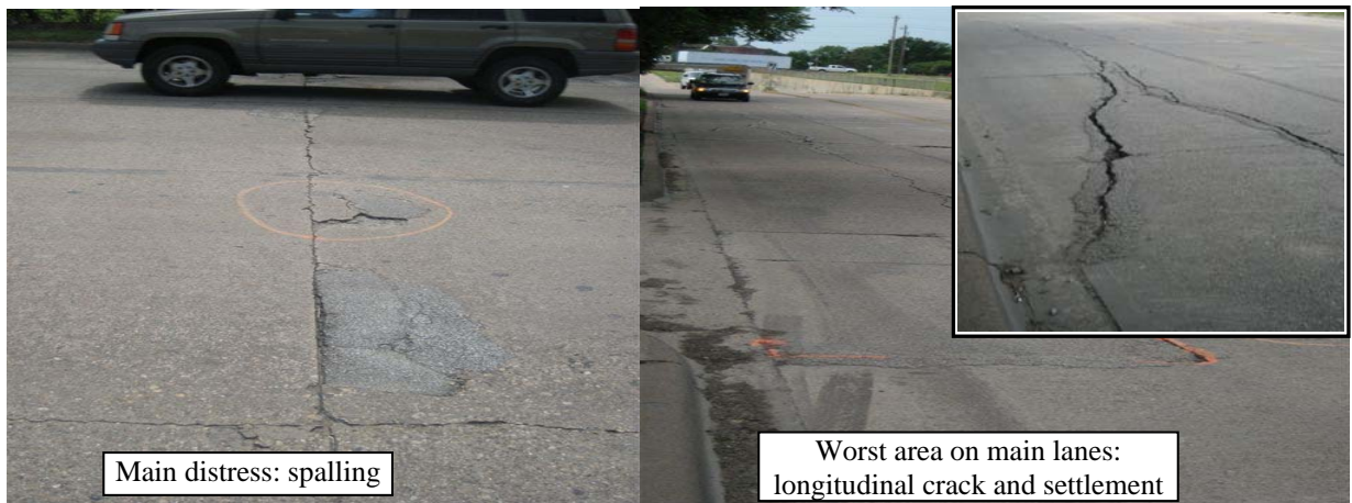
Figure 4. Observed Distresses on the Main Traffic Lanes, Pumphrey Drive, FTW.
