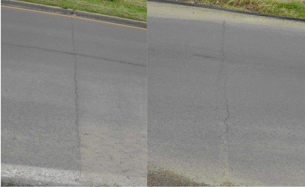
Figure 16. Examples of Transverse Reflective Cracking on Ramp R4.
