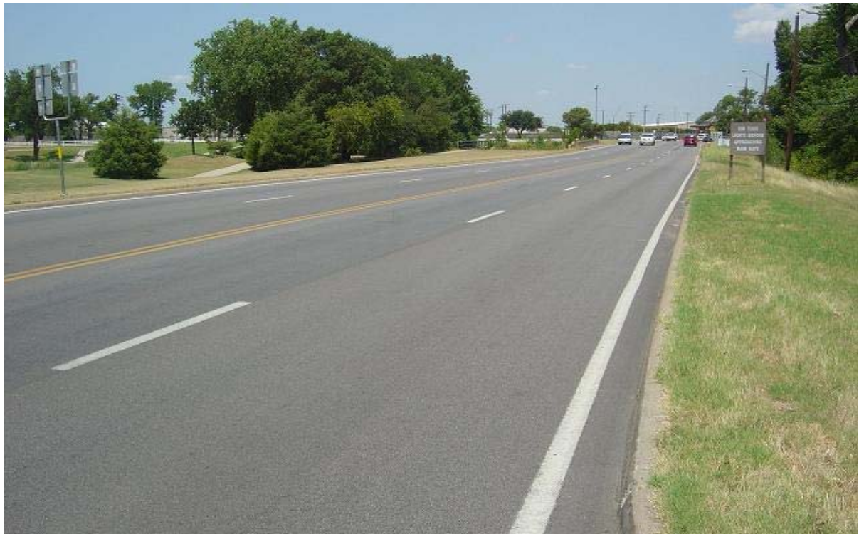
(14c). Overview of the Main Lanes in the Middle of the Project.
