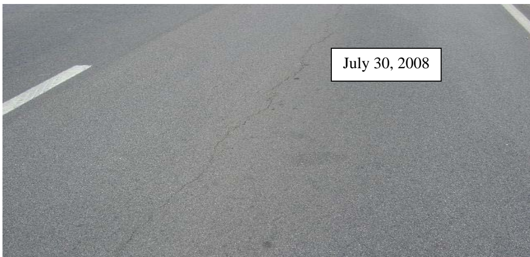
Figure 15. Longitudinal Cracking Manifesting in the Outside Northbound Main Lane toward the Naval Air Base Entrance.
