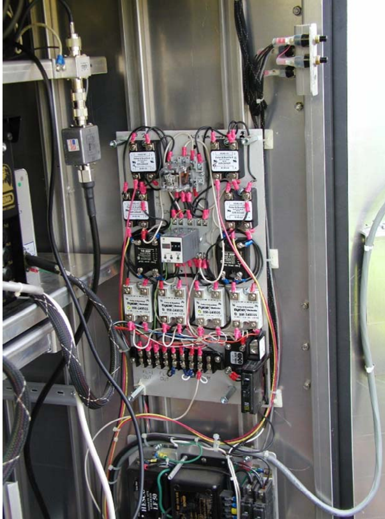
Figure 22. Flasher Panel Installed in a Cabinet.
