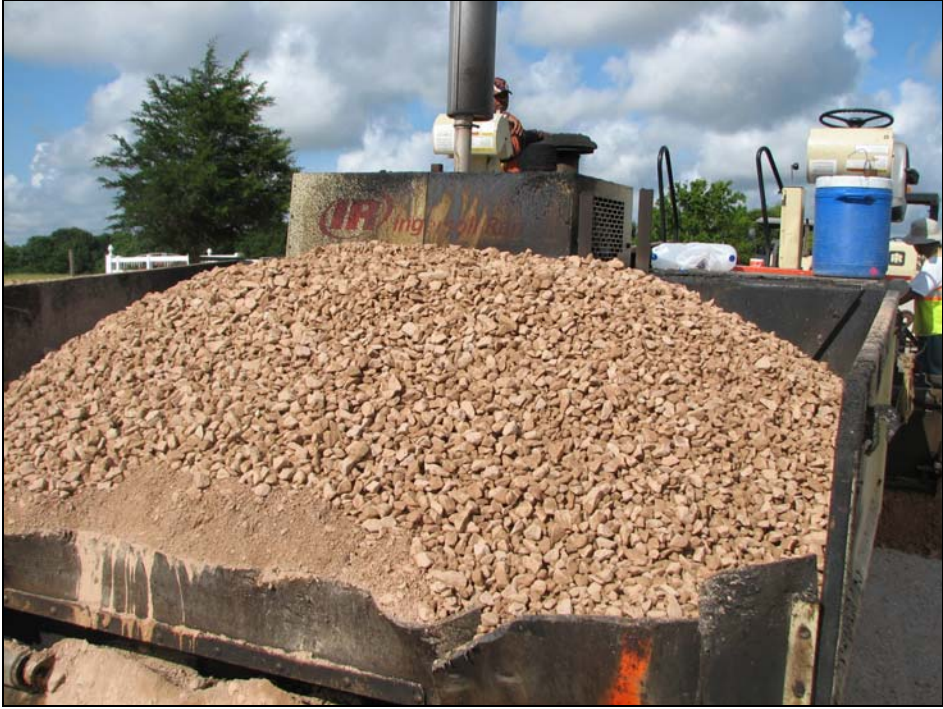
Figure 2.14. Segregation of Grade 4 Base in Paver Hopper.
