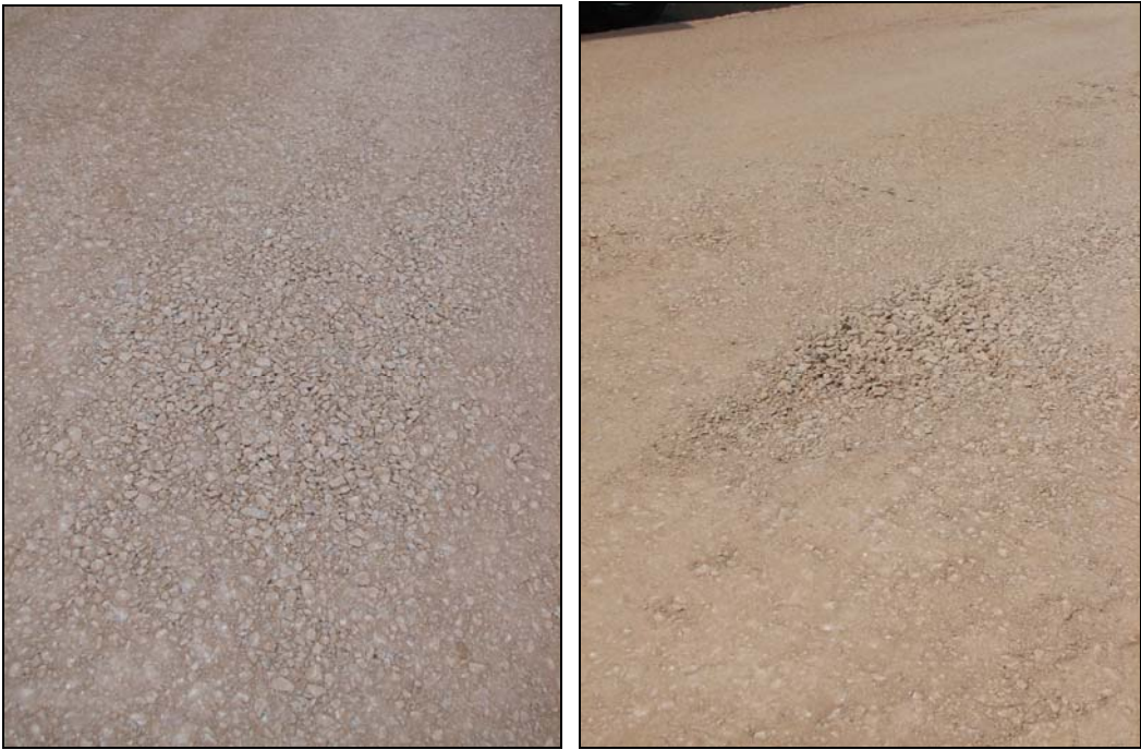
Figure 2.15. Segregation of Grade 4 Base after Placement.
