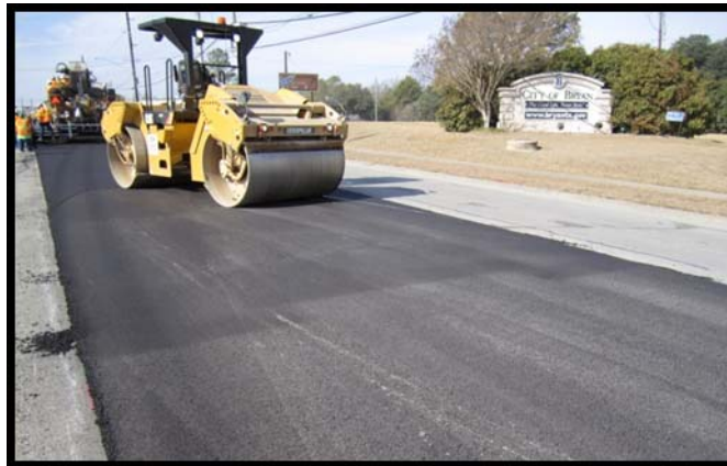
Figure 12. Pattern of Screed Left in Completed Mat due to Long Paver Stop.
