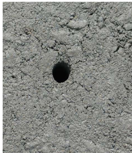
b) cracks induced before density test
