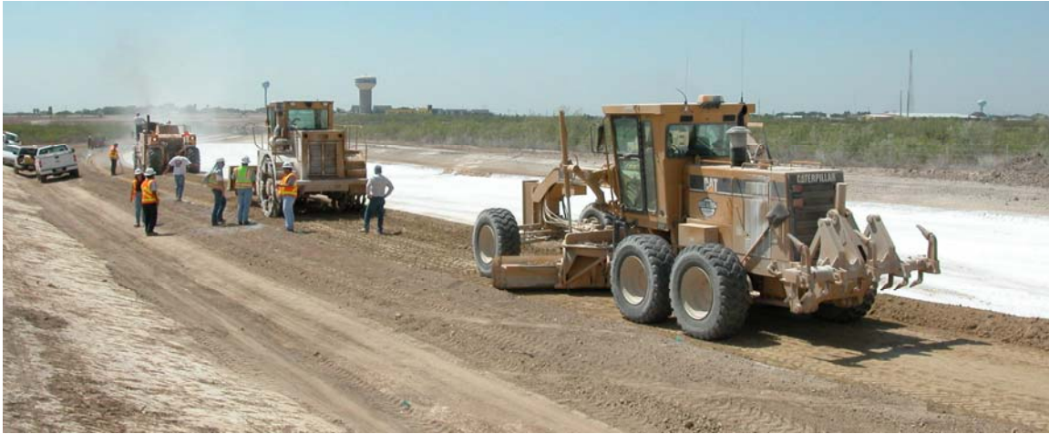
Figure 2.11. A Road Grader Was Used to Blade Off the Subgrade Following Compaction.
