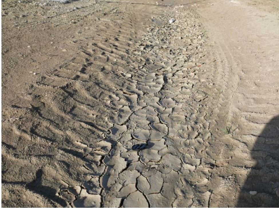
Figure 4.2. Drainage Ditch Adjacent to Second Street Shows Signs of Recent Rains.
