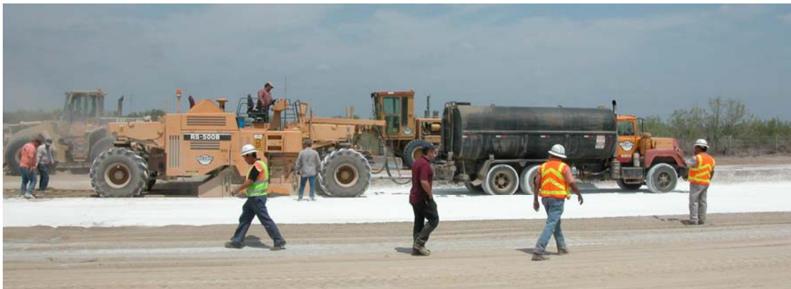
Figure 2.8. Addition of Water and Mixing of Lime into Subgrade in Eagle Pass.
