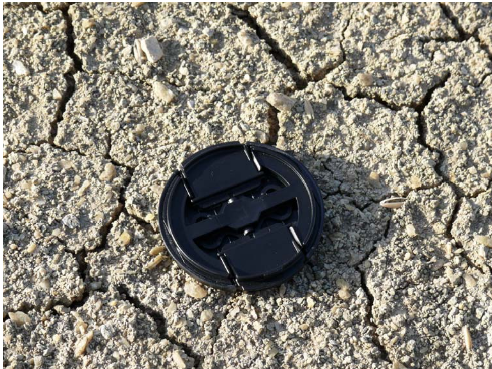
Figure 4.3. Gypsum Crystals Visible in Drainage Ditch Following Rains.
