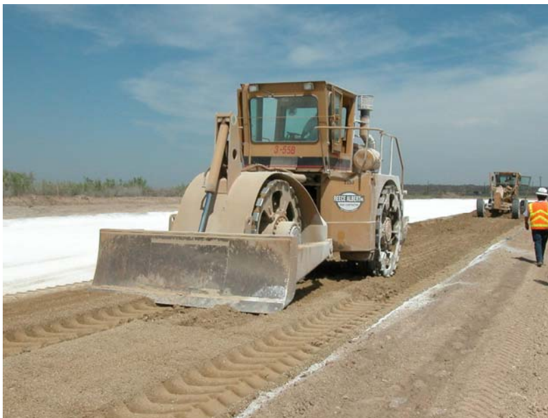
Figure 2.10. Padfoot Roller Used to Achieve Compaction Following the Mixing of Lime and Water.
