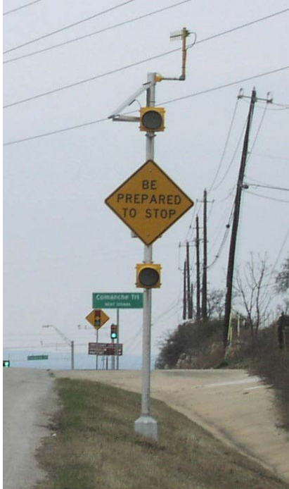
Antenna and Solar Panel
