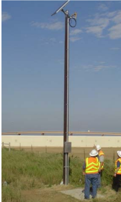
Antenna and Solar Panel
