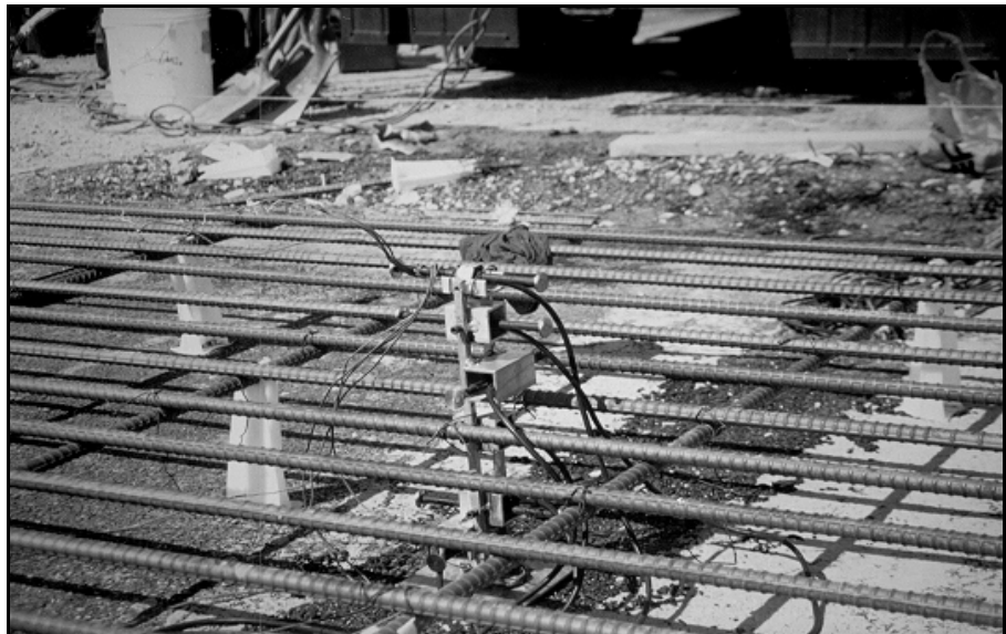
Figure 3.4. An Assembly of Five Concrete Gages Installed to Measure Concrete Strains in the Longitudinal and Transverse Directions at Different Depths.
