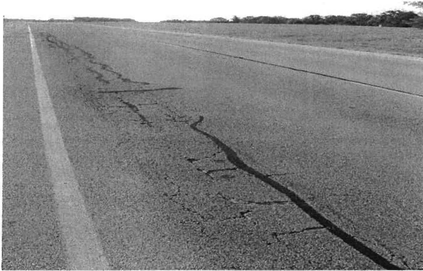
Figure 13. Structural Problems on SH 47.
