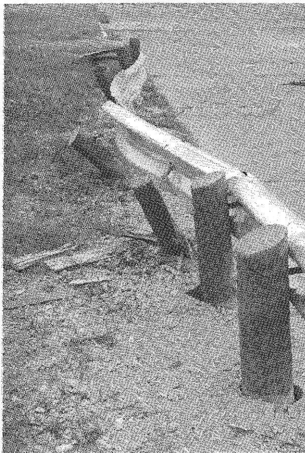
FIGURE 23. BARRIER DAMAGE AFTER TEST 3
