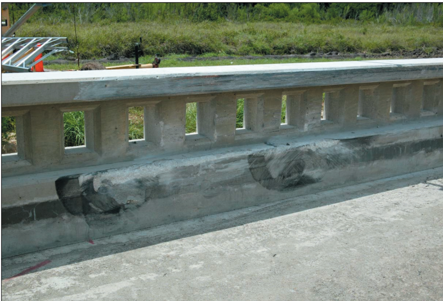
Damage to Texas F411 after pickup test.
