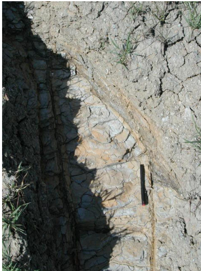
Figure 6. Gypsum Filled Fractures in the Eagle Ford Formation on U.S. 82.
