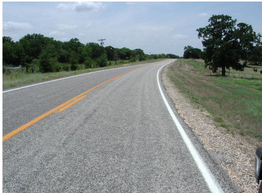
Figure 17. Condition of Second Geogrid Section on FM 1915 (No Distress after 3 Years in Service).
