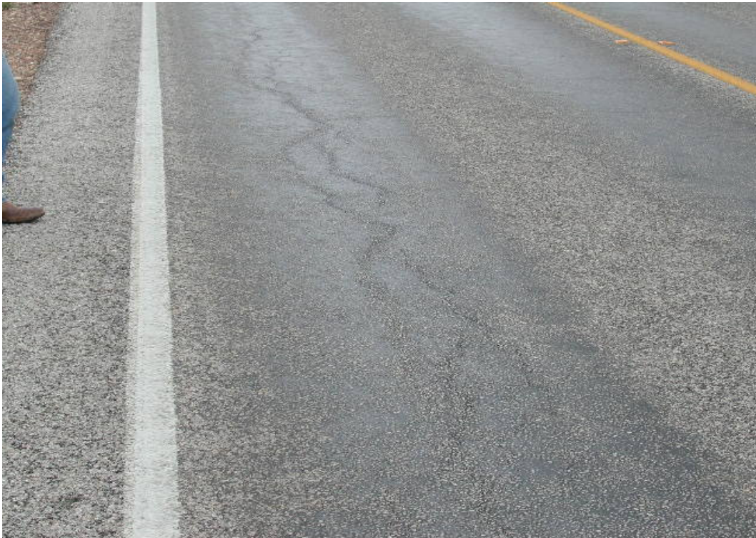
Figure 33. Wheel Path Cracking in the ATB Section.
