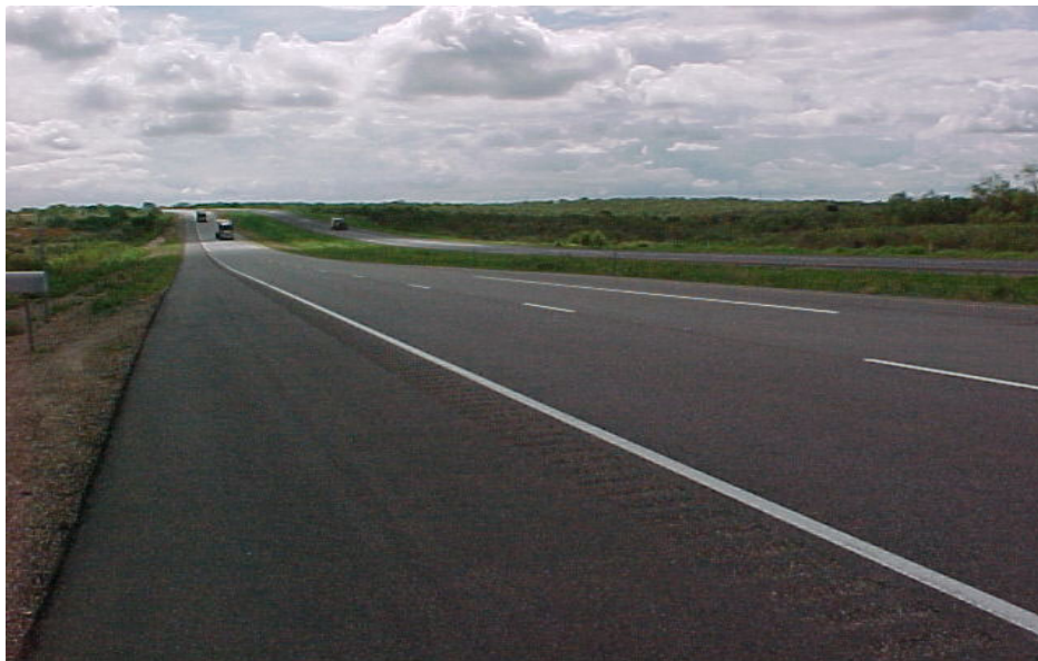
Figure 24. US 287 near TRM 216 (10 inch Fly Ash Base (6% FA), 2 inch HMA Constructed Summer 1998, Heavy Traffic, Excellent Condition).
