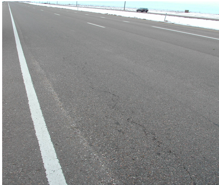
Figure 30. Section 5 US 87 SB Dalhart to Hartley (Last overlay 2 years old). Emulsion stabilization (2%). FWD indicated that the stabilized layer is weak. Structural damage apparent after 7 years.
