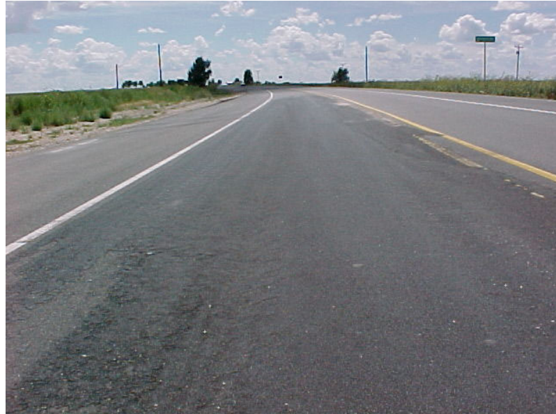
Figure 29. Section 1 SH 207 Hutchinson County – Cement/Fly Ash Base. Patched area, initial problems relating to slippage between the base and surface.
