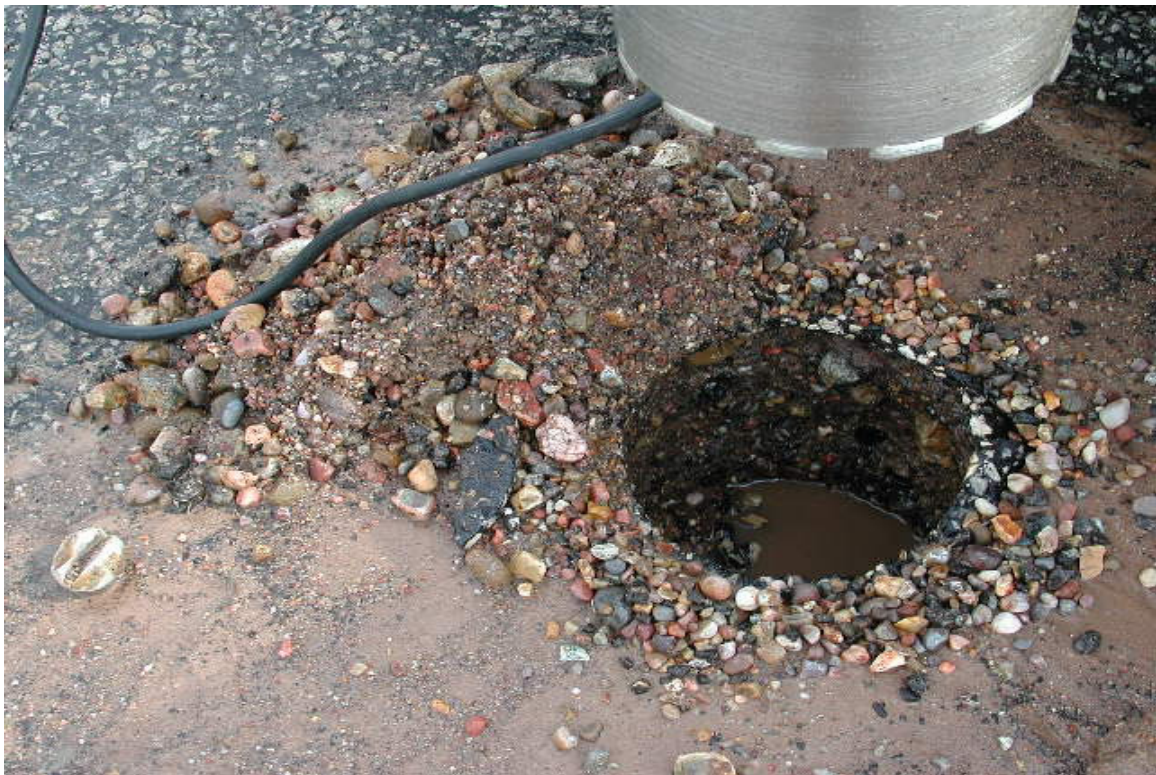
Figure 38. Coring Emulsified Base (No Evidence of Base Stabilization).
