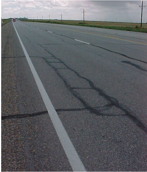
Figure 27. Loop 335 NB CTB Structural Damage.
