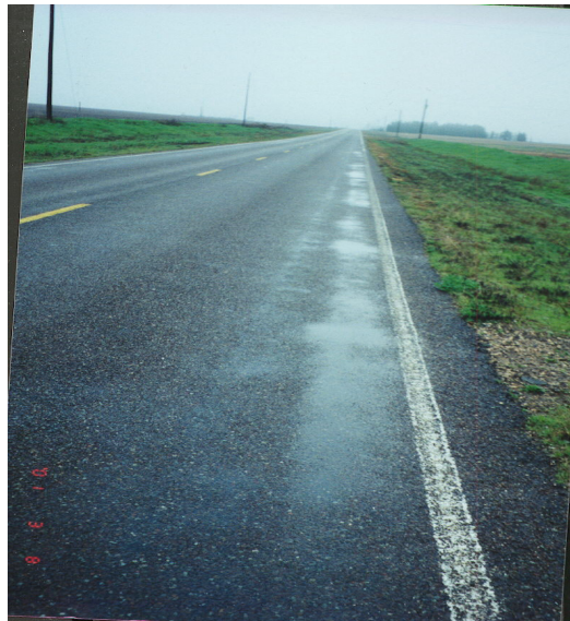
Figure 23. Minor Rutting on FM 399 Garza County.
