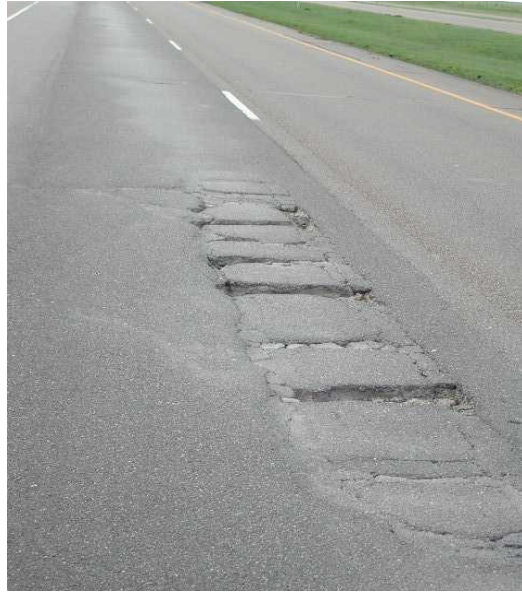
Figure 28. IH 40 EB CTB Structural Failure.
