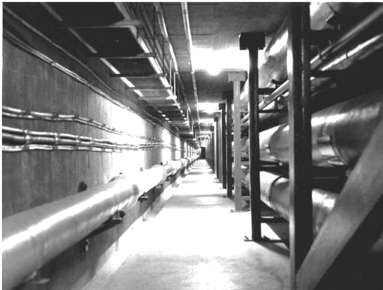
Figure 2-3. Steam Tunnel with Utilities (13).
