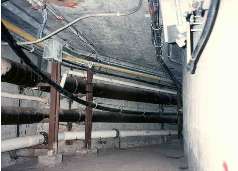
Figure 2-2. Example of Steam Tunnel with Utilities (13).
