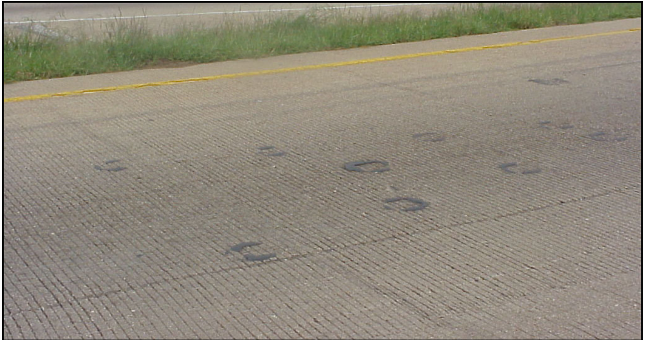
Figure 5. Wrong-Way Arrow with all Raised Pavement Markers Missing.
