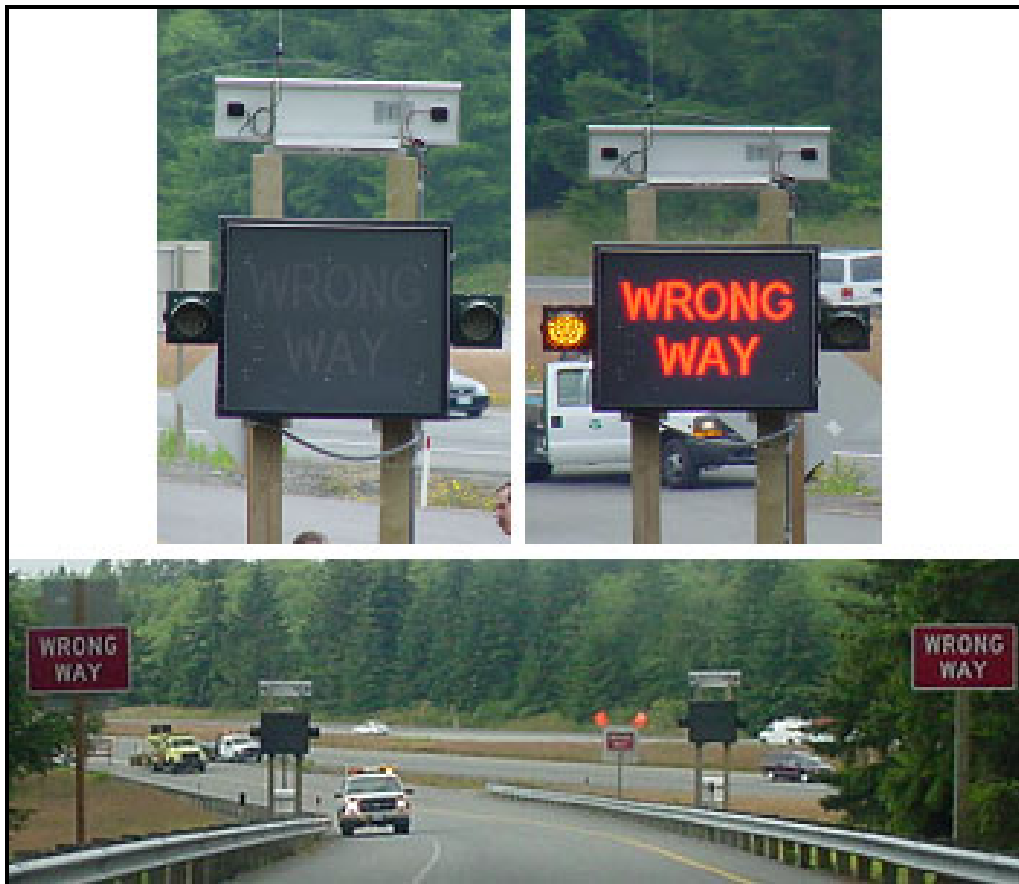
Figure 34. Washington State Wrong-Way ITS System on an Exit Ramp.
