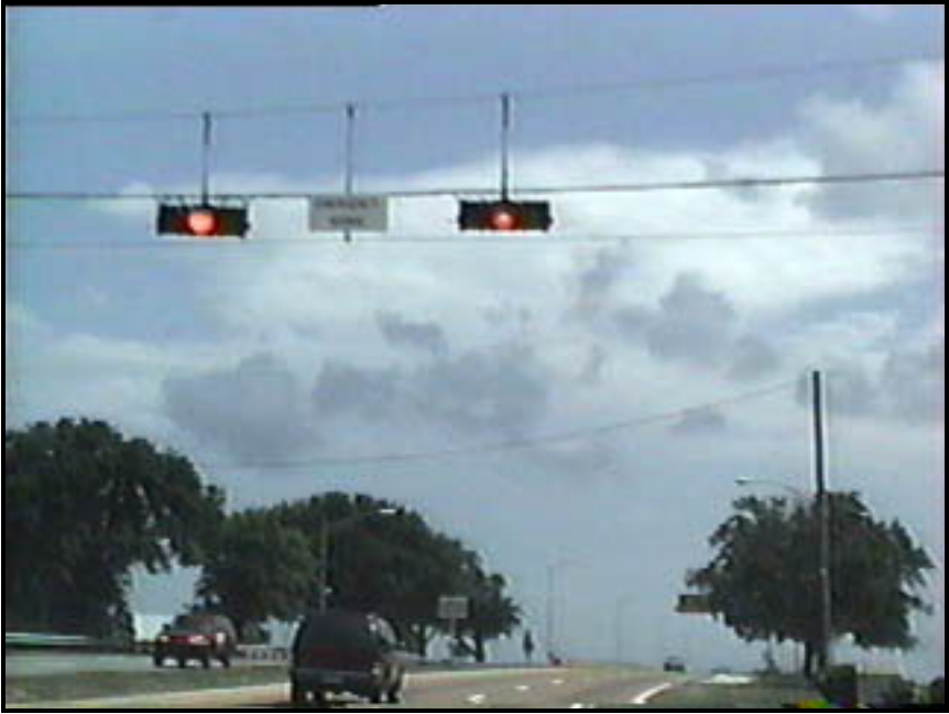
Figure 37. Florida Bridge Wrong-Way Signal System.
