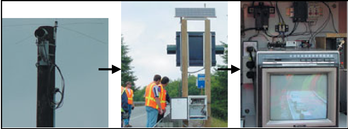
Figure 5. Video Monitoring System on Exit Ramp in Washington State (5).
