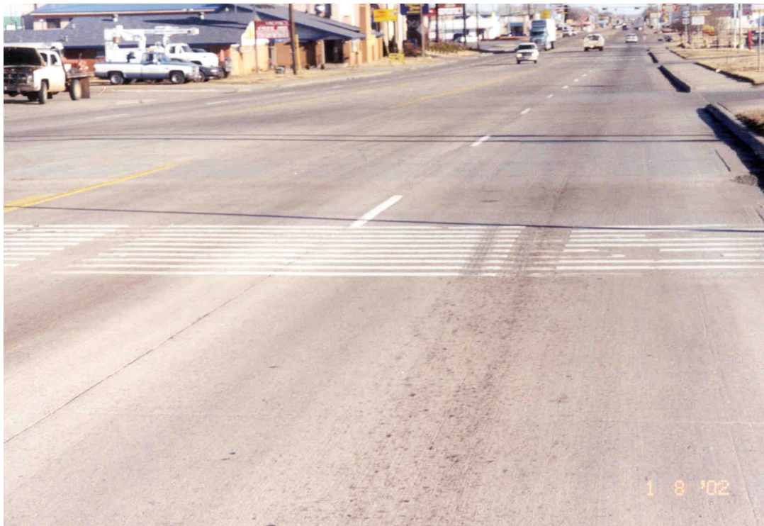
Figure 12. View of Approach Rumble Strips.
