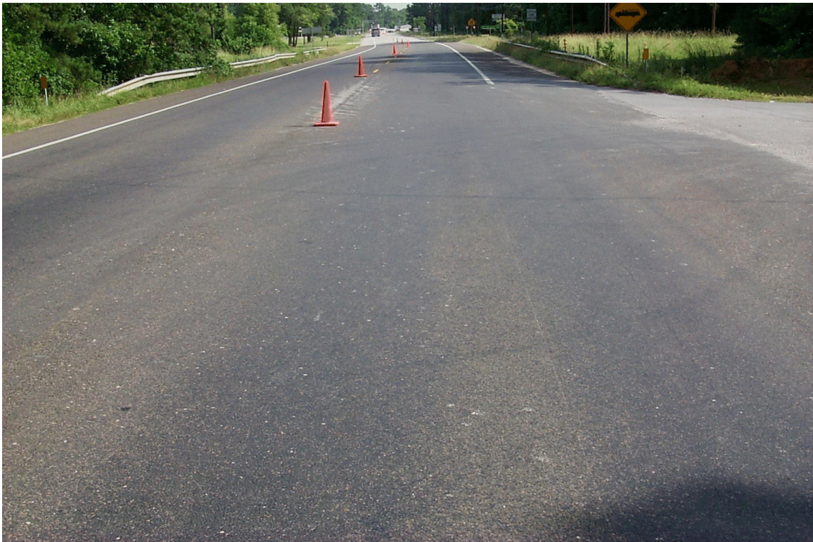
Picture 1. High Severity Bleeding.
