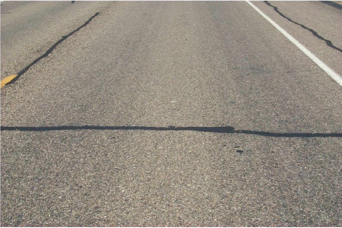
Picture 2. Low Severity Bleeding.
