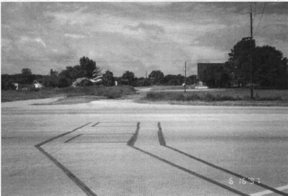
Figure 2-2. Temporary Inductive Loop and Piezoelectric Sensors.
